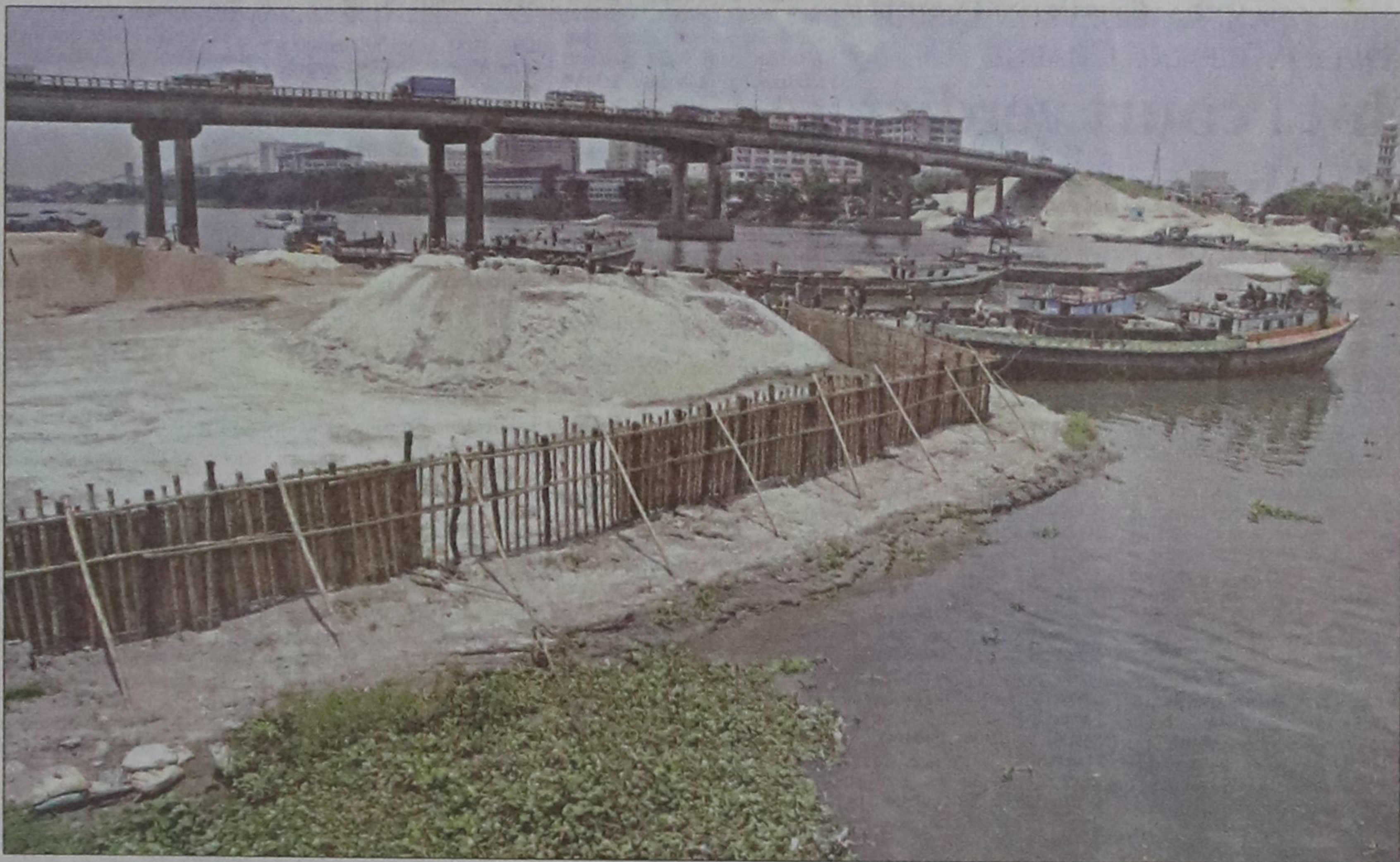
Sand traders erect a fence and fill up a section of the Shitalakhya to stock sand. The photo was taken near the Kanchpur Bridge.
