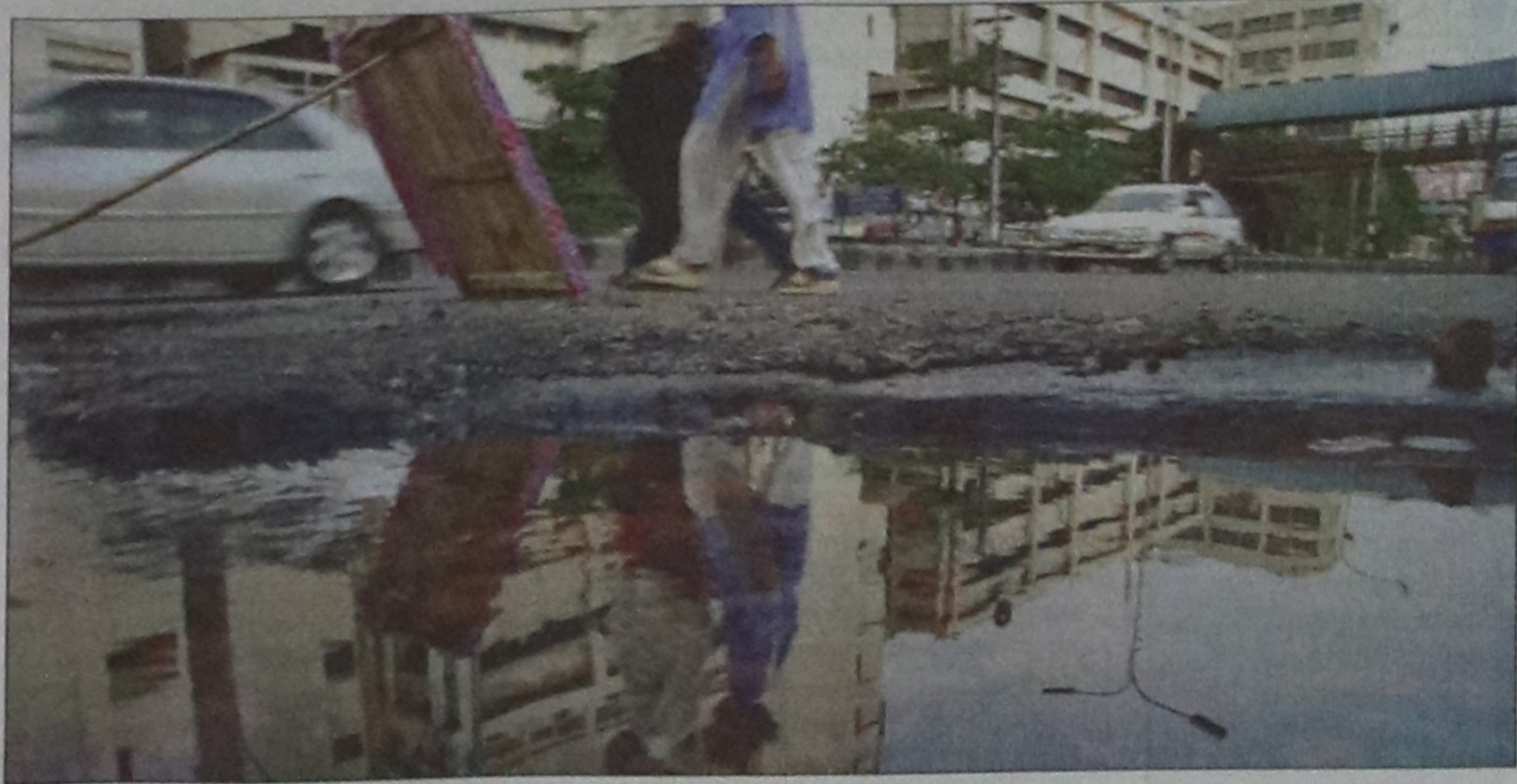
Water coming out of underground Wasa pipeline in front of Bangabandhu Sheikh Mujib Medical University at Shahabagh in the city yesterday causes suffering to pedestrians, but the authorities appear to have turned a blind eye. PHOTO: STAR
