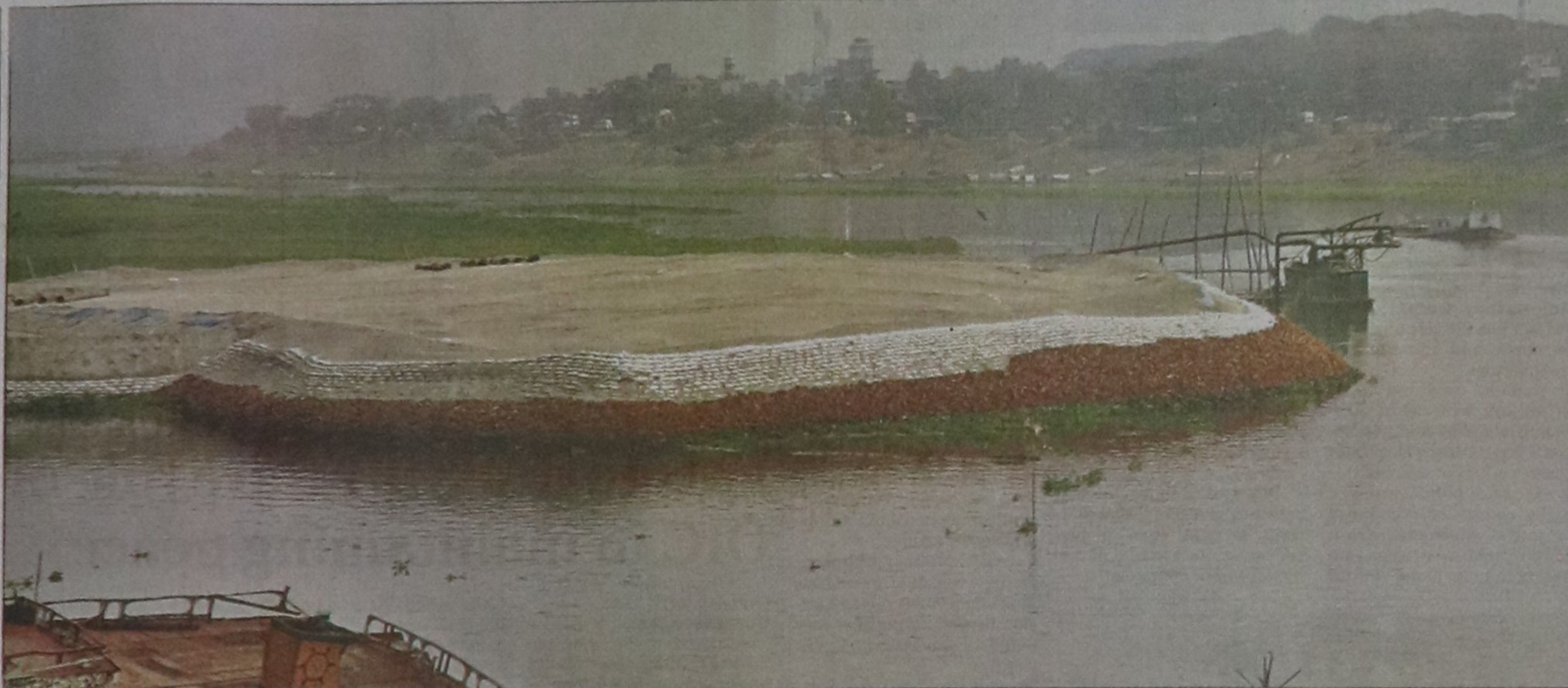
A vested quarter fills up a portion of the Turag near Sinnirtek to sell plots to people. The photo was taken from Mirpur flood embankment across the river.
