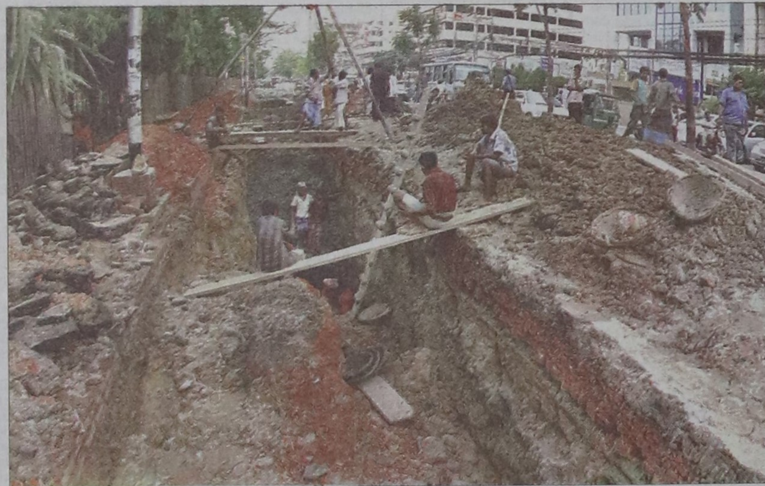
Dhaka Water Supply and Sewerage Authority (Wasa) is setting up sewerage pipes near Panthakunja Park blocking one lane of CR Dutta Road to the suffering of city dwellers.
