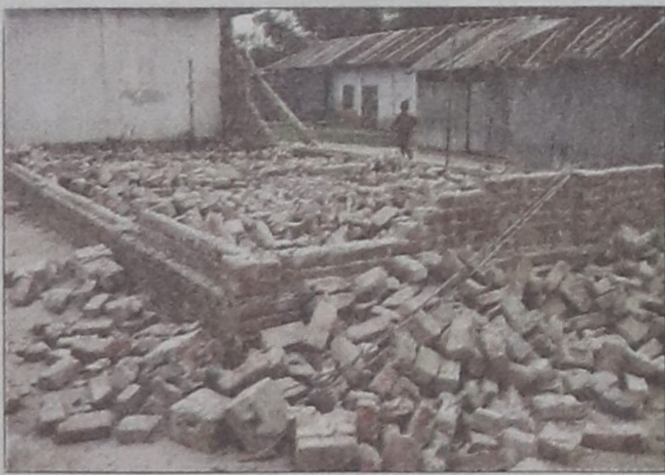
A room of Balapukur High School in Aditmari upazila collapsed on Saturday night, only five months after its construction.
