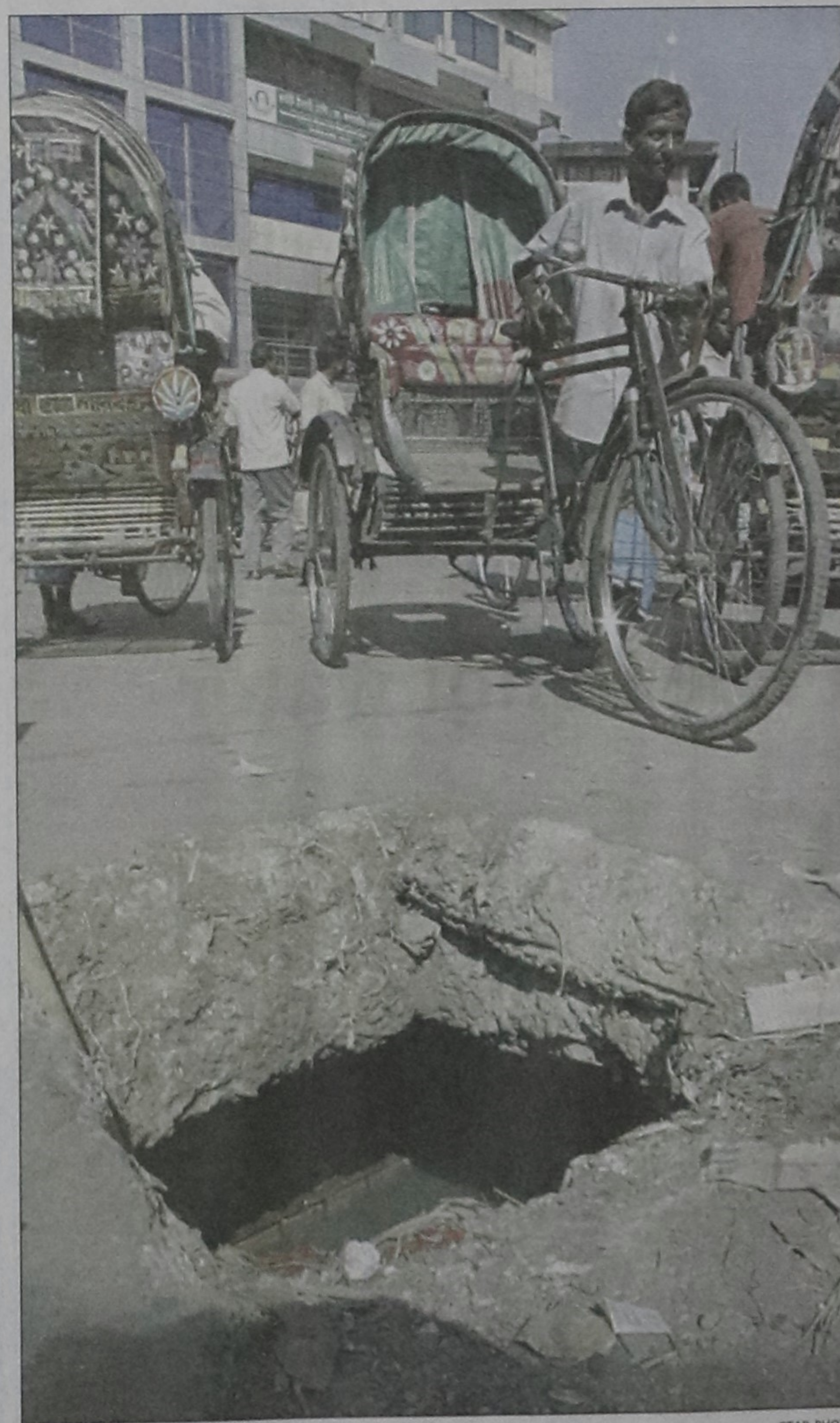
A broken manhole on the busy Reazuddin Bazar Road poses danger to commuters and pedestrians, but the authorities appear to remain indifferent. The photo was taken on Tuesday.
