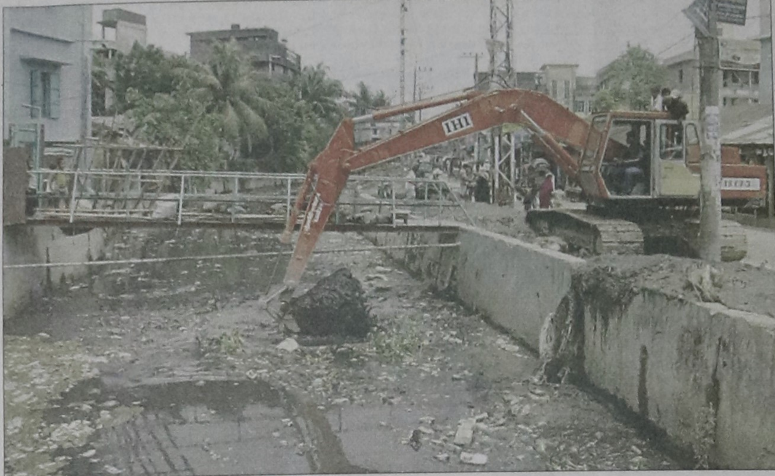
Chittagong City Corporation (CCC) excavates the Chaktai canal ahead of rainy season. The photo was taken from Dhunirpul area of Chawkbazar on Monday.
