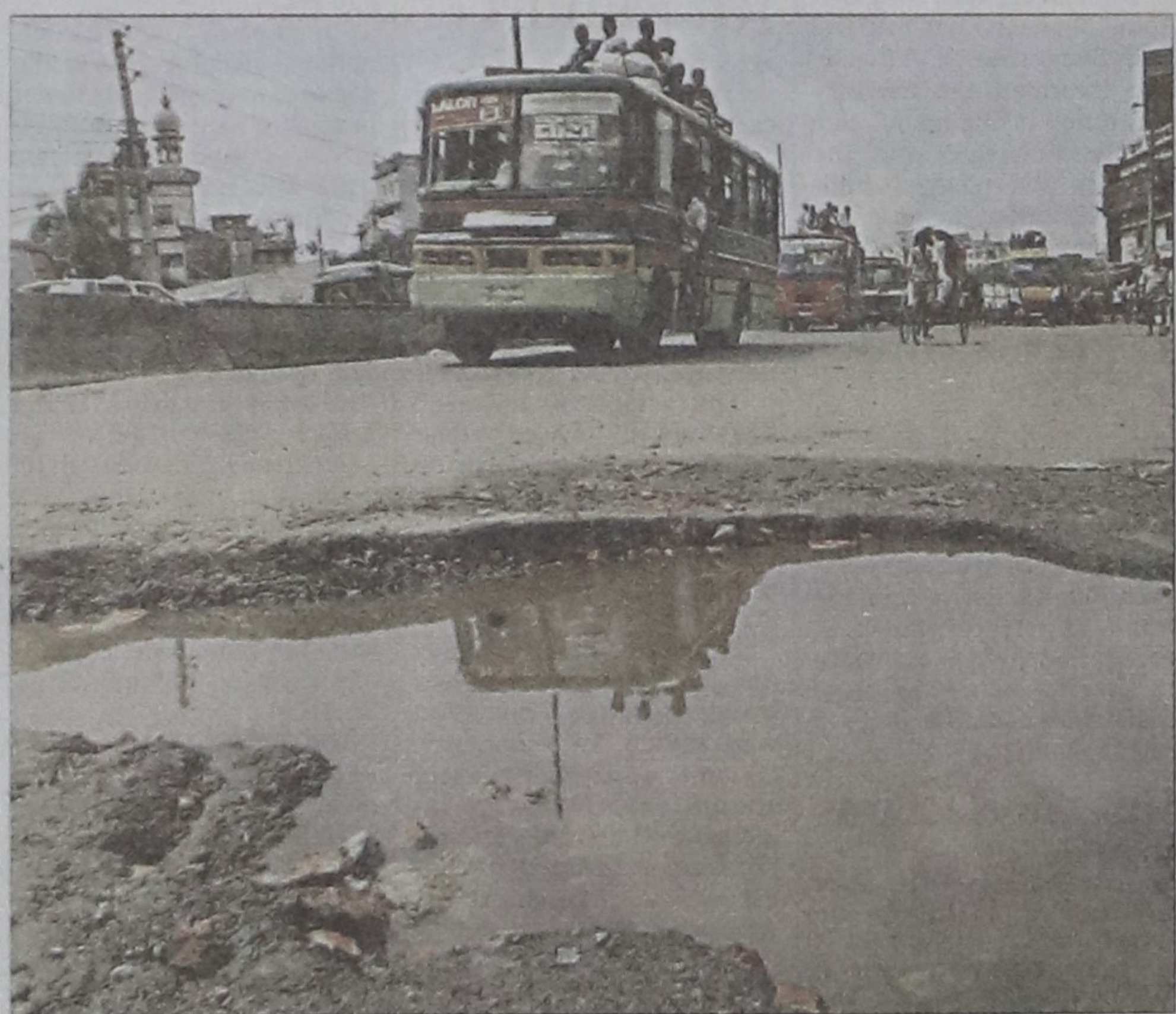
This large pothole on the street in front of Sayedabad Bus Terminal has been causing mishaps almost every day for the last six months with the authorities concerned turning a blind eye.
