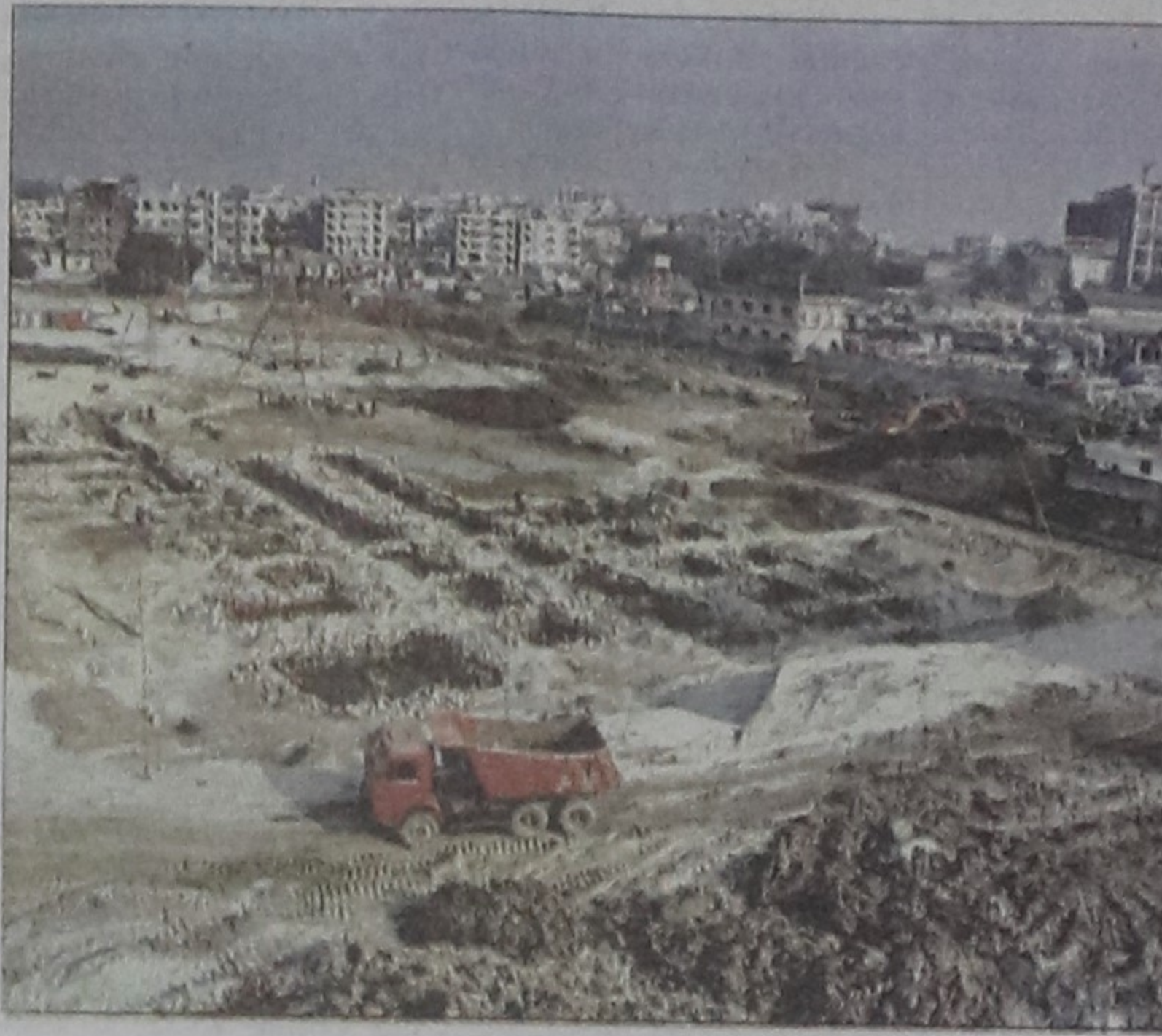
The construction work of the wholesale kitchen market in Mohakhali, left, and the one in Jatrabari, right, in the capital goes on slowly and is on the verge of closure due to increasing cost and lack of additional funds.
