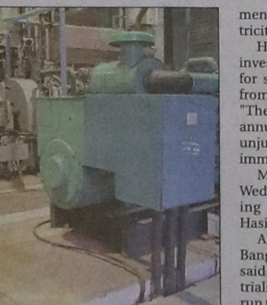
A captive power plant at an industrial unit to cope with frequent outages.
