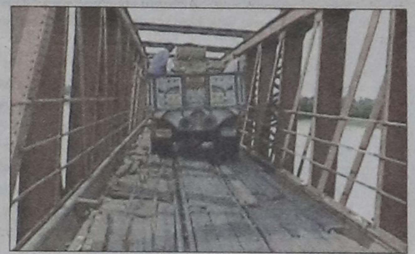
Run-down Teesta bridge in Lalmonirhat.
