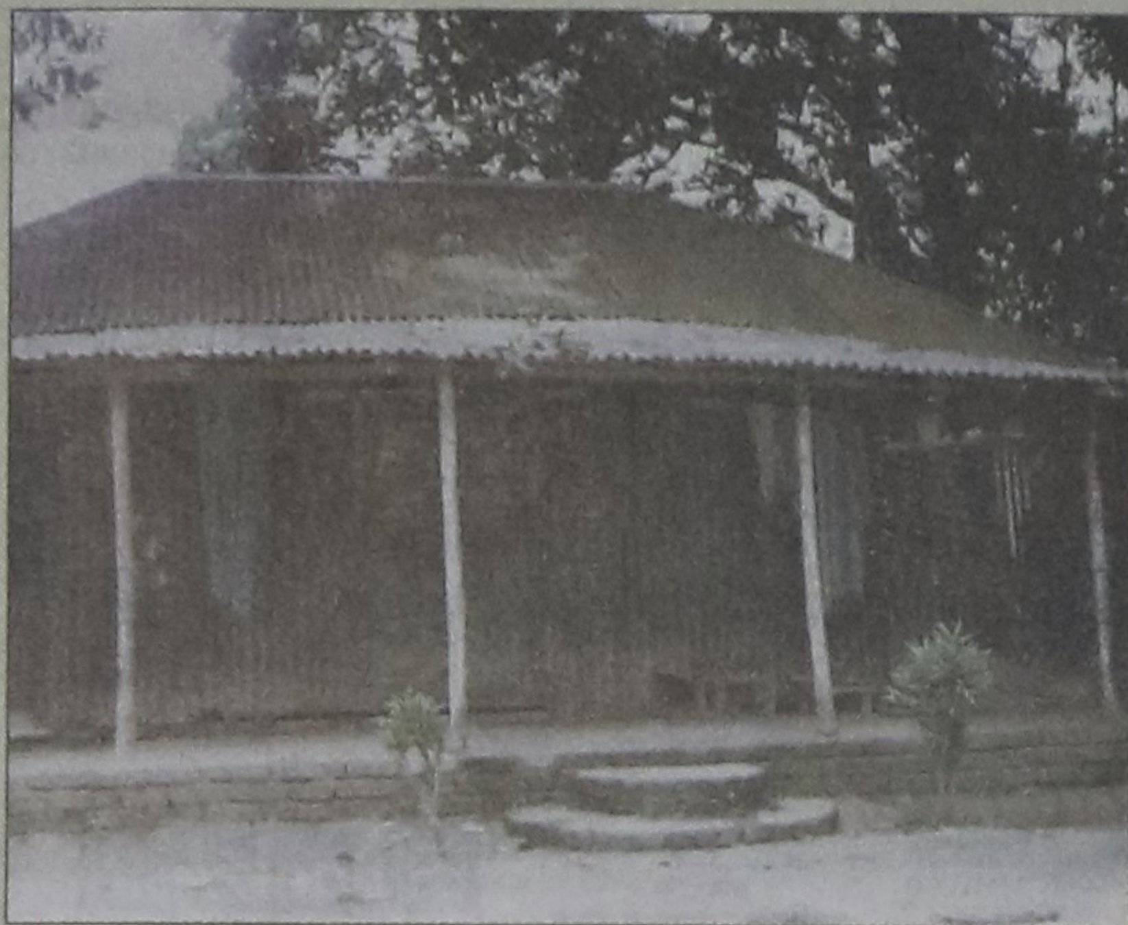
Mostafa's ancestral home is in a state of disrepair.
