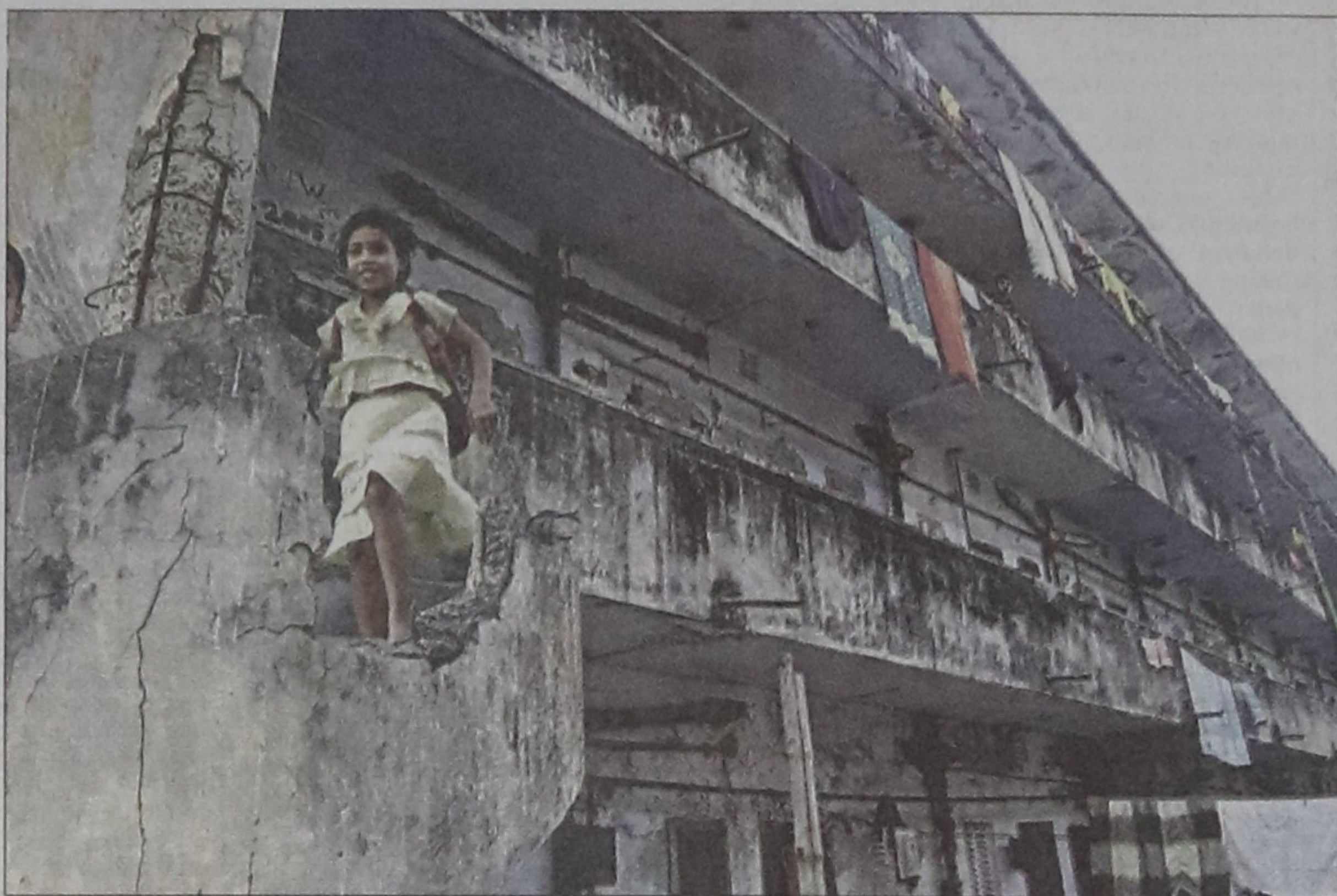
A child climbs down the stairs of a dilapidated AGB colony building that was declared unsafe for living five years ago.
