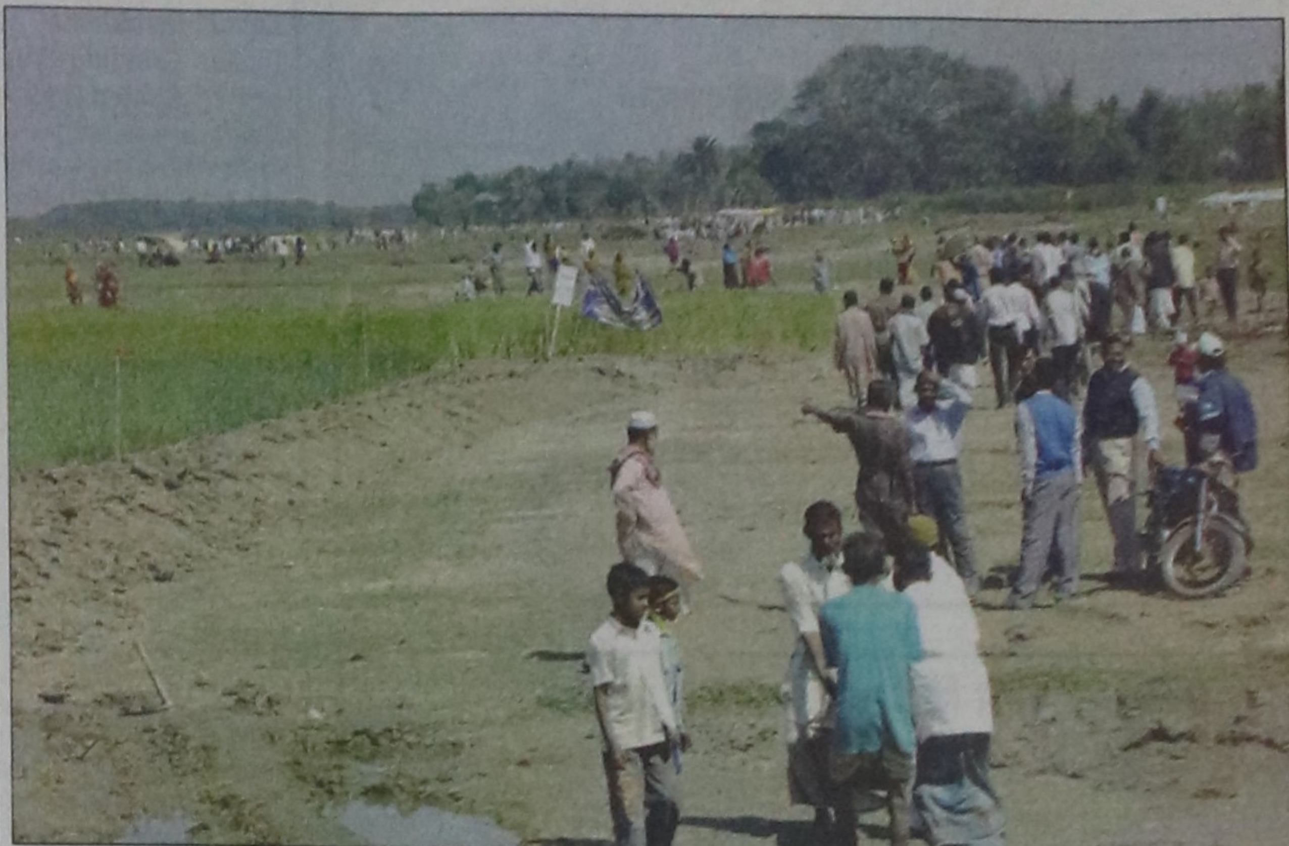
UNITY IS STRENGTH: Villagers rendering voluntary service to construct a five-kilometre road from Notun Kahela to Dimukhi Bazar in Warshi union in Mirzapur in Tangail under 'Shouhardo' project of CARE Bangladesh. Five thousand villagers including women and students of 19 villages joined hands to complete the work by today. About 40,000 villagers would be benefited on completion of the road.
