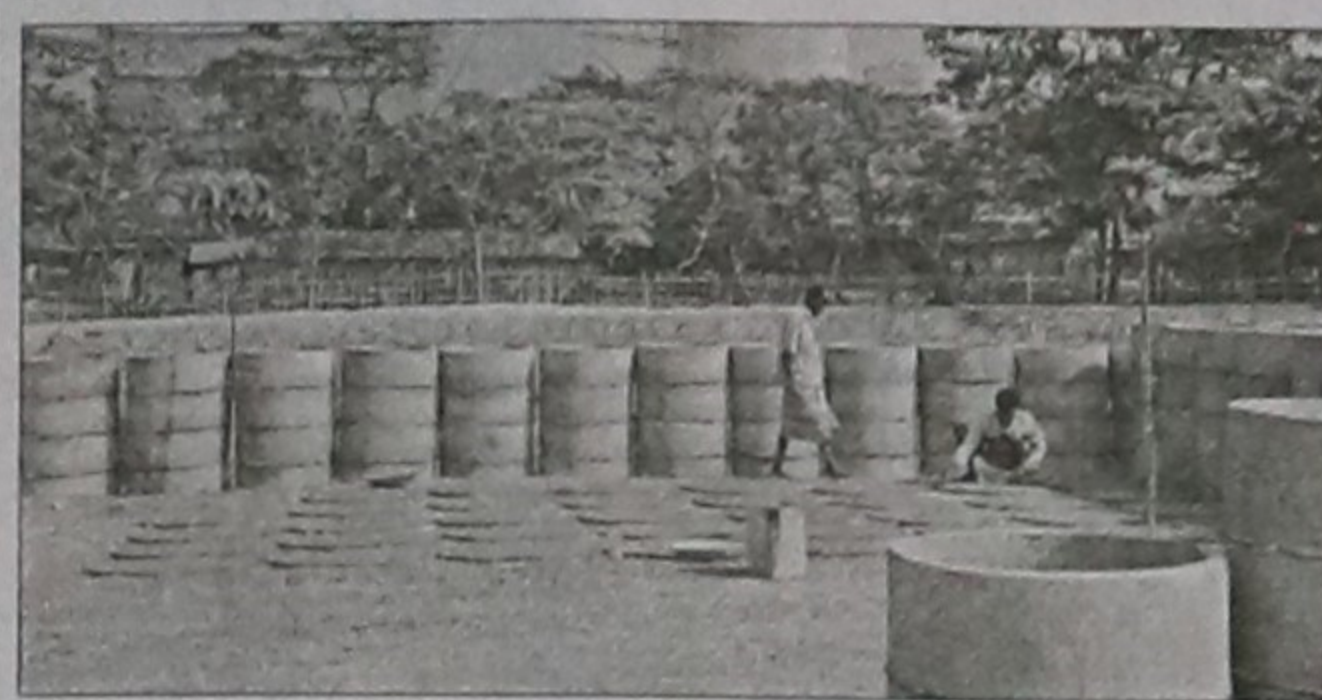
Masons prepare sanitation wares beside the Lafarge Surma Cement Plant in Chhatak.
