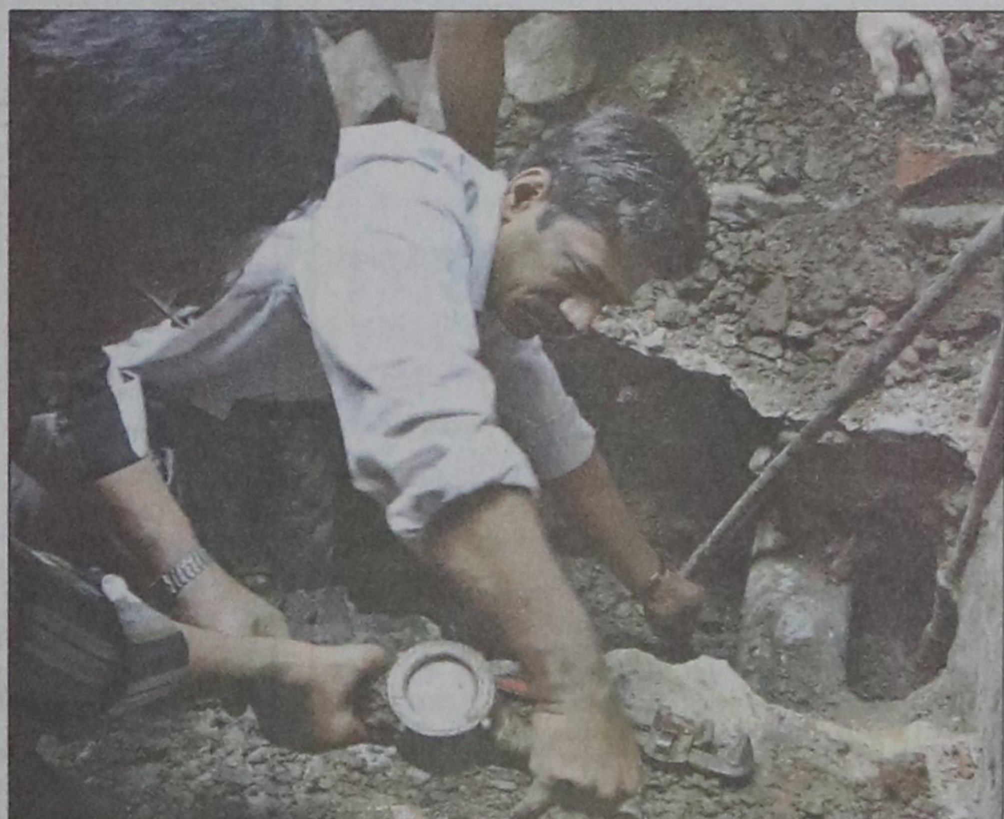
Workers of Dhaka Water Supply and Sewerage Authority (Wasa) disconnect the connection of a bill defaulter at Azimpur in the city yesterday for failing to pay outstanding bills. PHOTO: STAR
