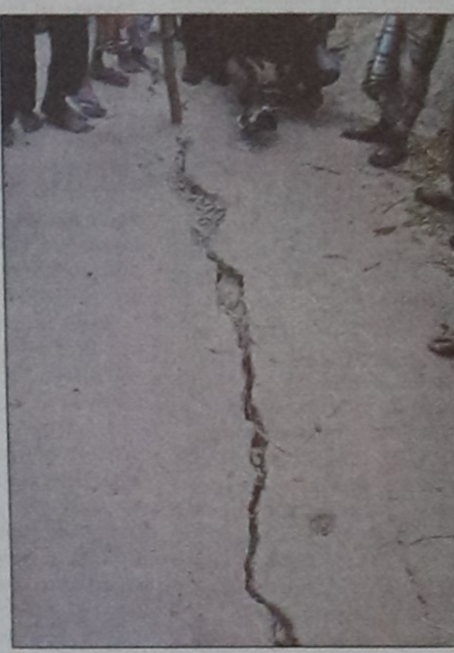
Cracks appear on a village road near the Barapukuria Coalmine. Some of the cracks are 20-40m long.
