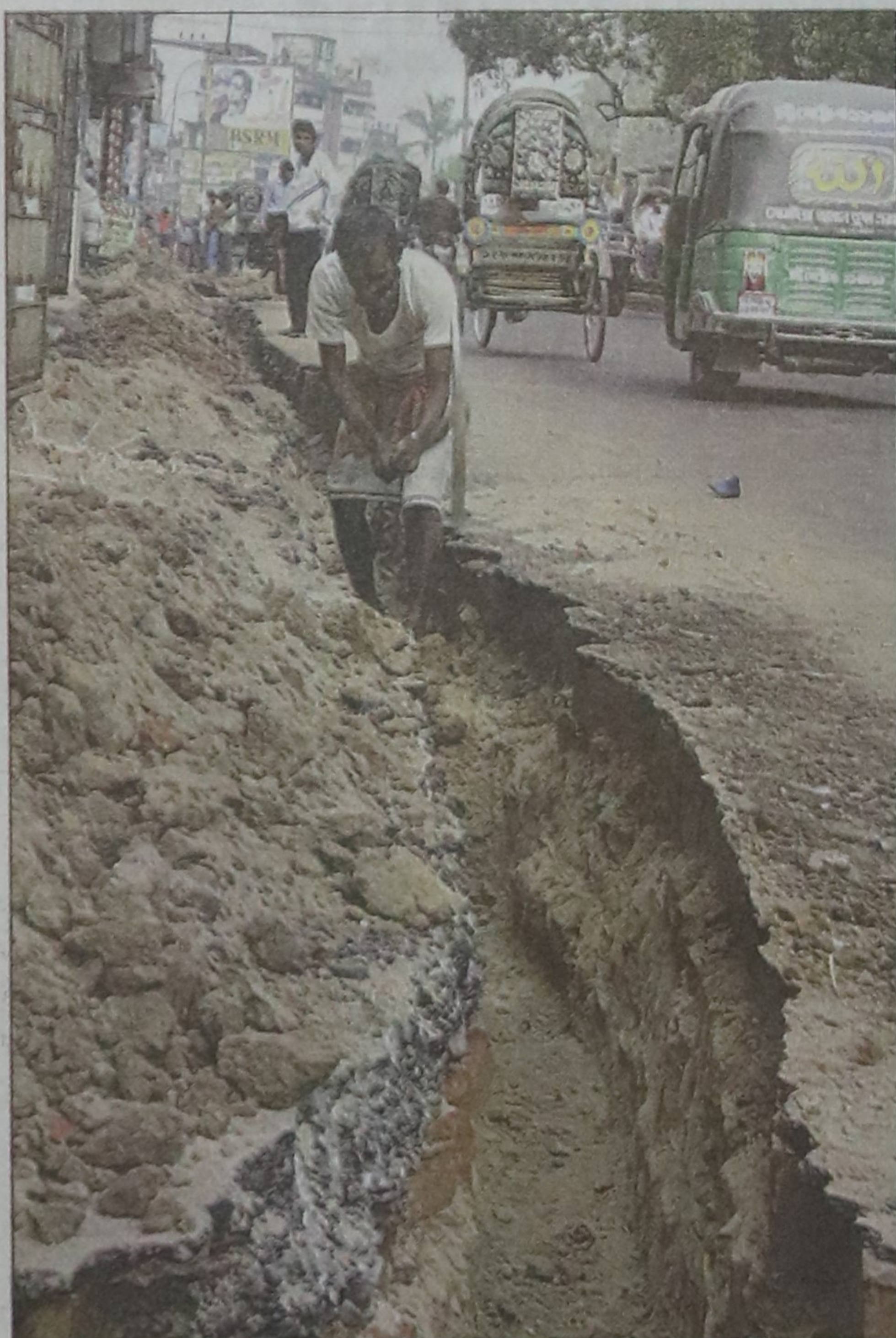
Different roads in the port city are being dug again for expansion of mobile phone network that were renovated a few months ago, causing serious gridlock and sufferings to the pedestrians and locals. The photo was taken from DC Hill area on Sunday.
