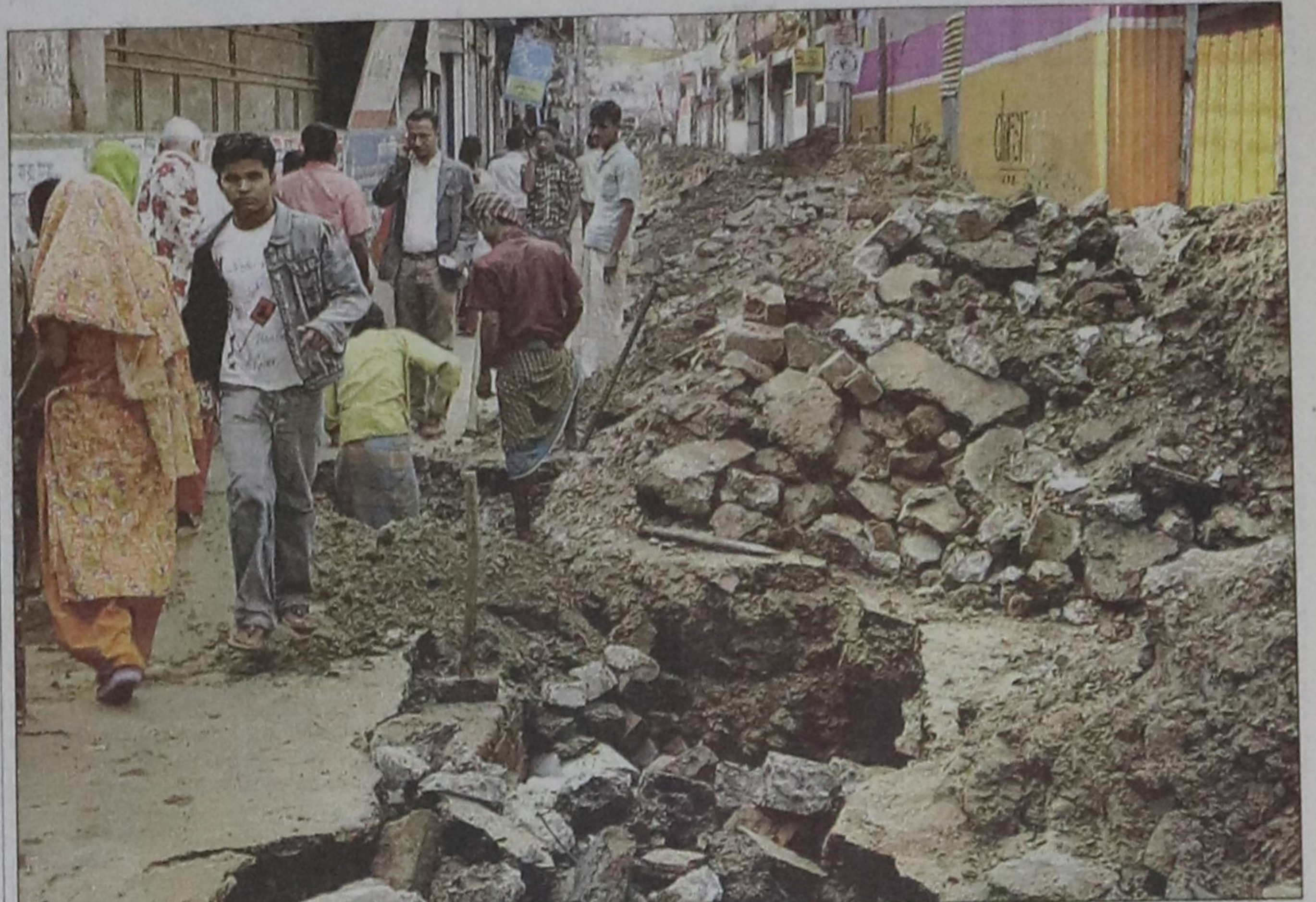
The work for laying of sewerage pipe has been going on at Free School Street at Kathalagan in the city for over a month, causing suffering to pedestrians as well as local residents. PHOTO: STAR
