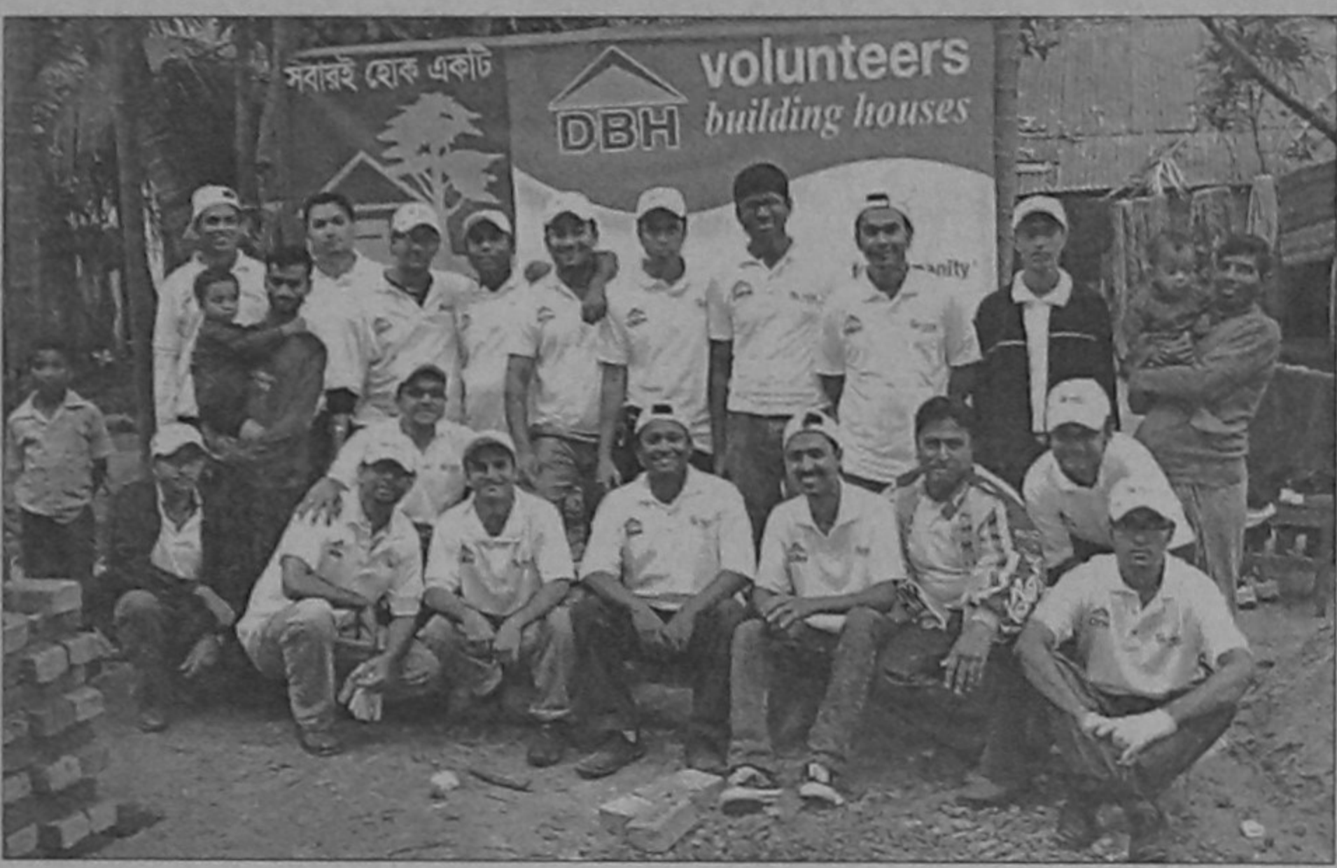
Employees of Delta Brac Housing Finance Corporation Ltd (DBH) take part in 'volunteers- sponsorship home build activities' launched by the Habitat for Humanity International Bangladesh (HFHIB) for low-income people at Kaliganj in Dhaka on Saturday.
