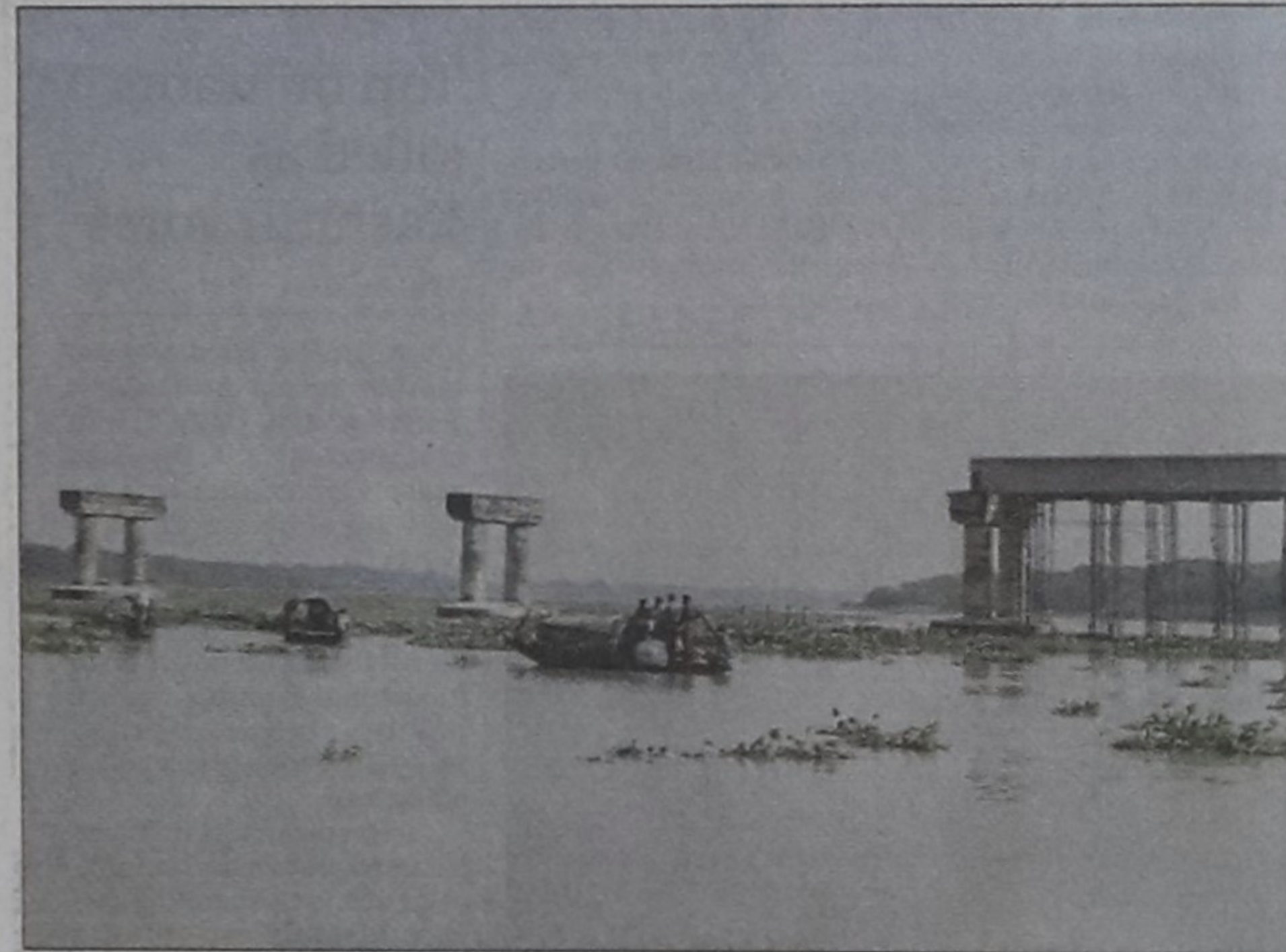
Work of Taltali Bridge on the Taltali River in Barisal still remains incomplete although three former lawmakers promised several times to construct the bridge before elections.
