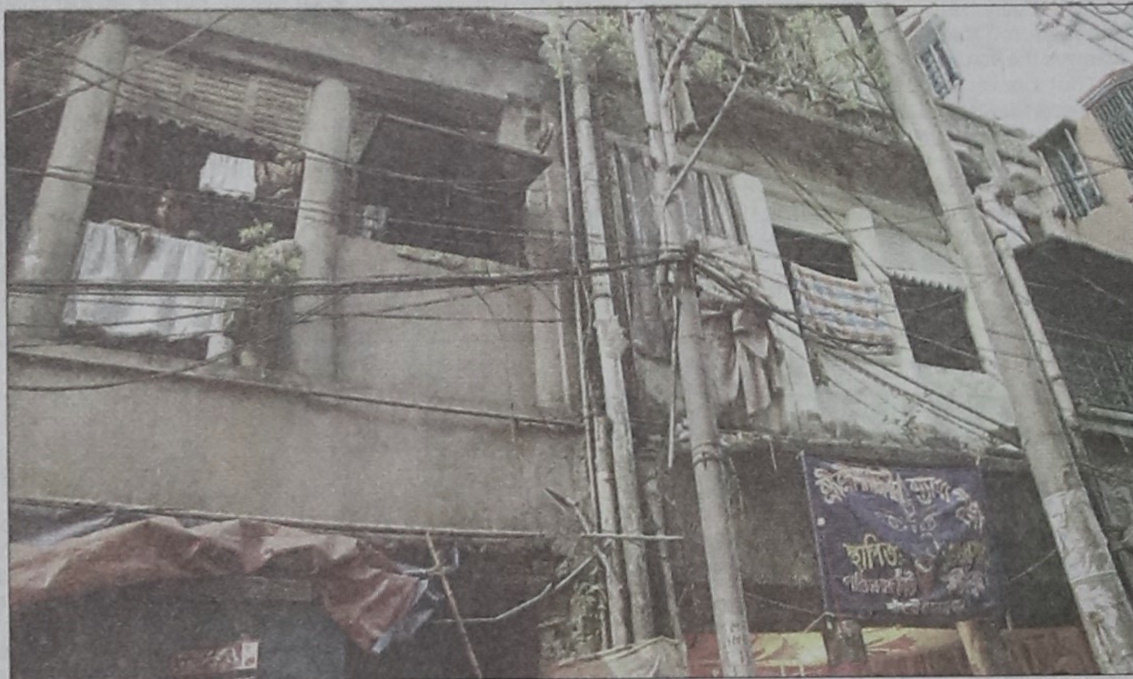
Residents at Shankhari Bazar are living in dilapidated buildings risking their lives.
