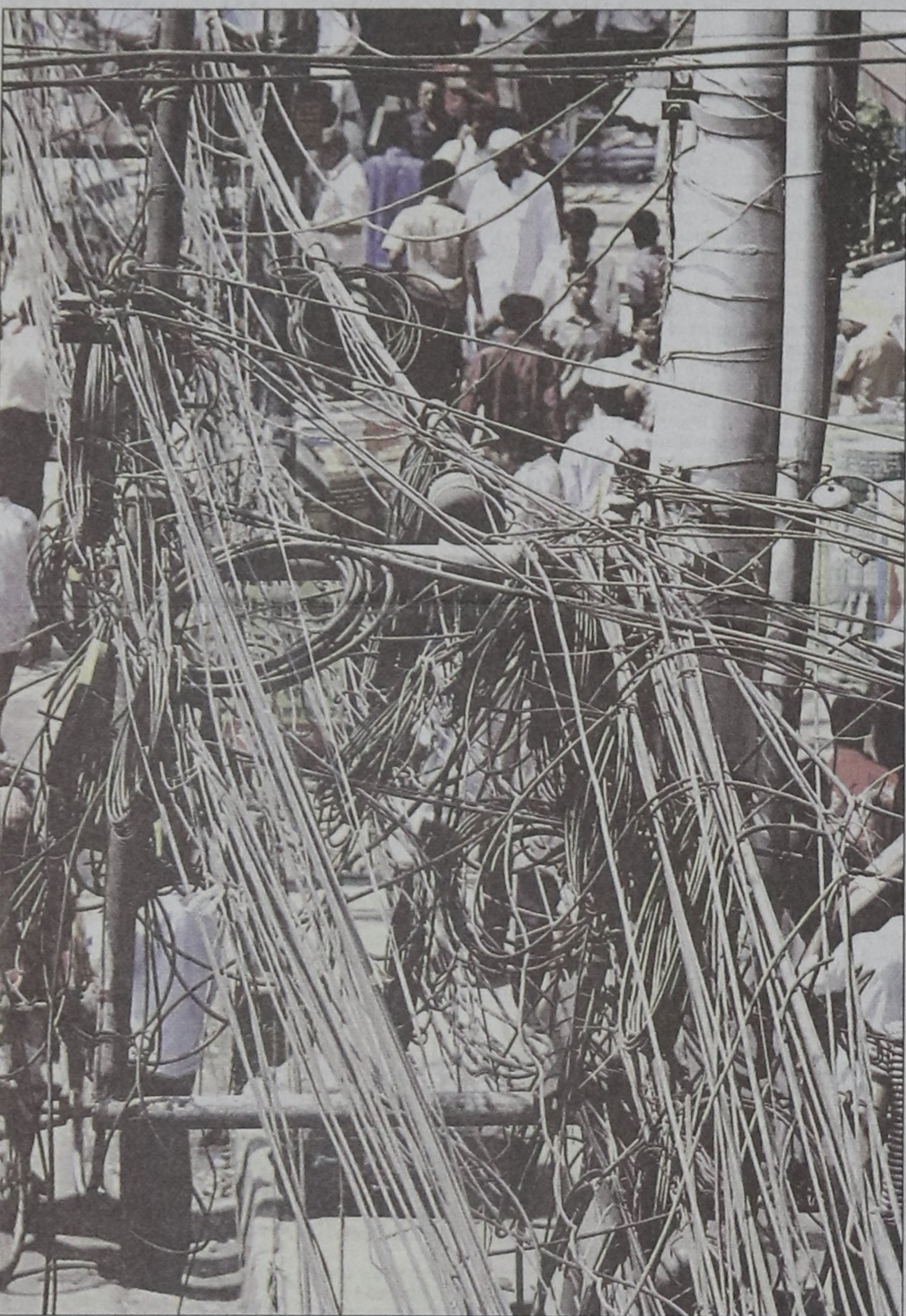
Electric lines, cable TV cables, telephone wires and cables of Internet service providers tangled on a government pole at Paltan in the capital. PHOTO: STAR
