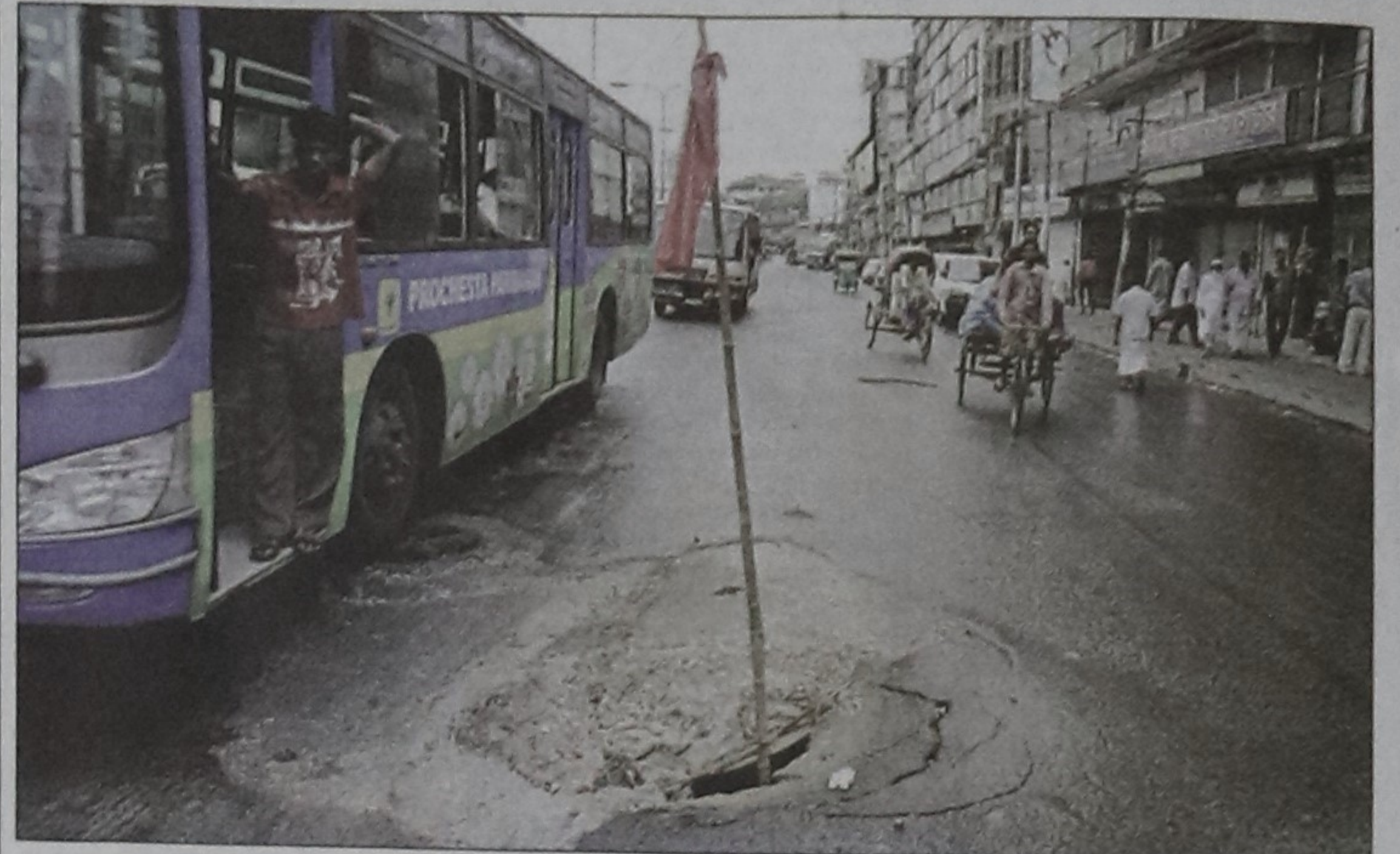
Locals place a bamboo pole inside a gaping hole on the road between Mouchak intersection and Malibagh level crossing to warn vehicles of the danger as authorities concerned are yet to fix it. PHOTO: STAR
