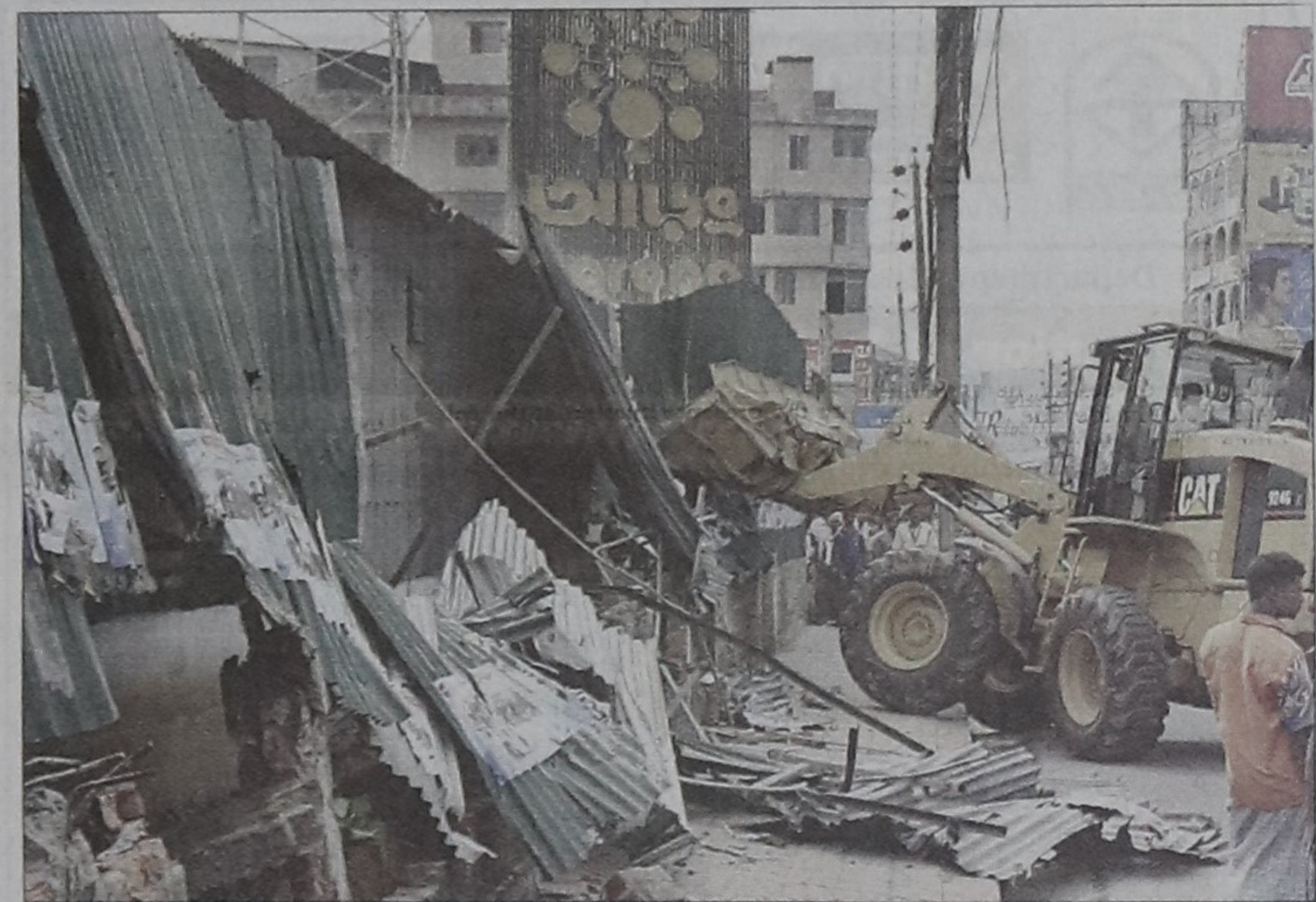
Rajuk bulldozes unauthorised structures along Tejgaon-Gulshan link road under Hatirjheel-Begunbari Integrated Development Project in the city yesterday.
