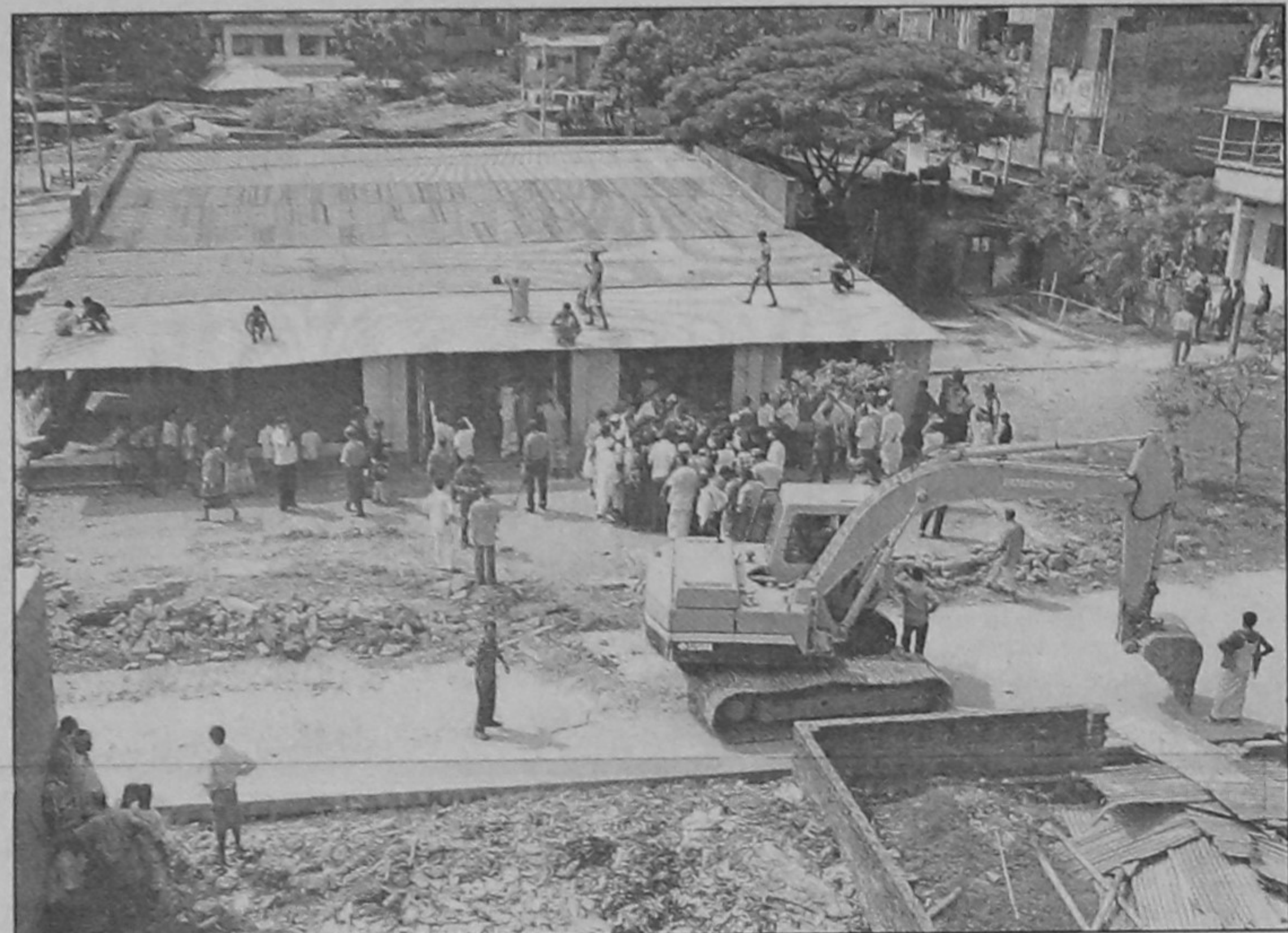
Public Works Department authorities dismantle illegal structures at Mirpur in the city yesterday.
