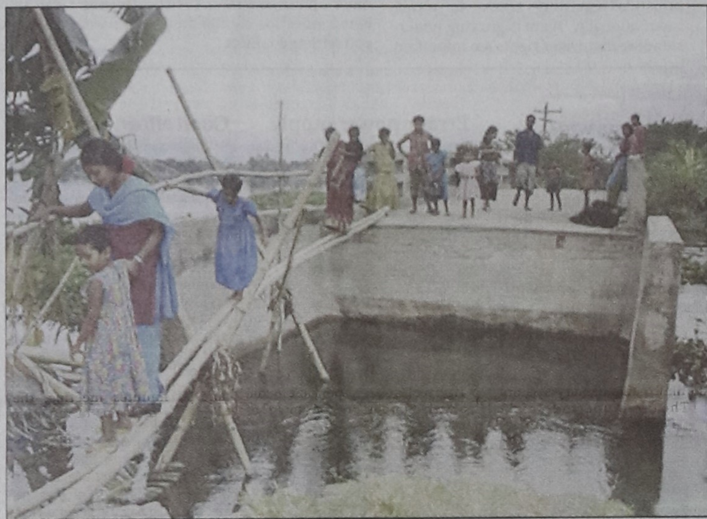
Cautious walk on a bamboo structure to cross Shurgram Bridge on Ramdia-Boltali road in Gopalganj as the approach road has remained unrepaired after the recent flood washed it away.
