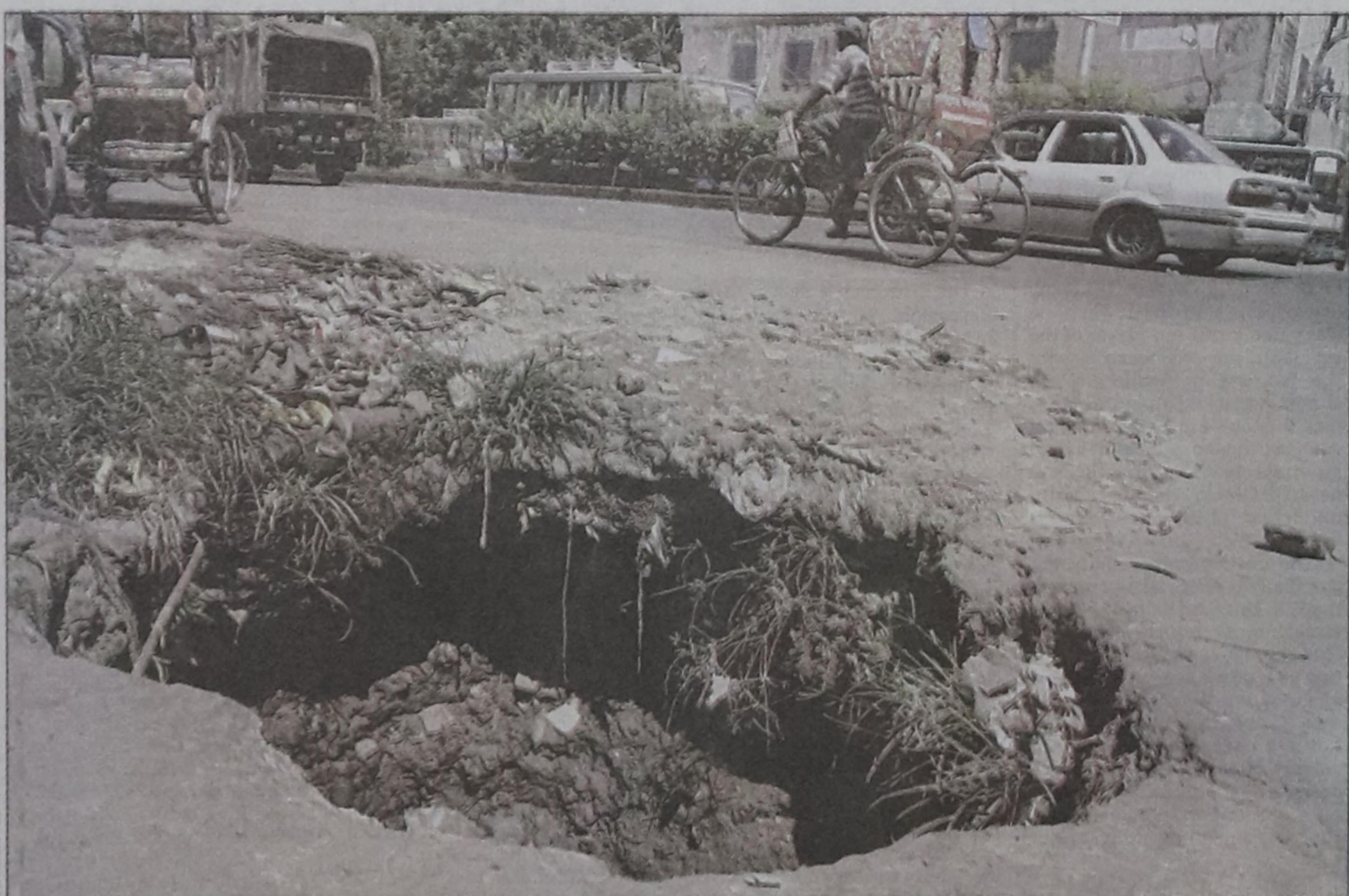
A portion of the Harun Mollah Road caved in turning it into a death trap for pedestrians in Mirpur Pallabi 12. The gaping hole lies open for weeks but the authorities are yet to take any step to repair it.
