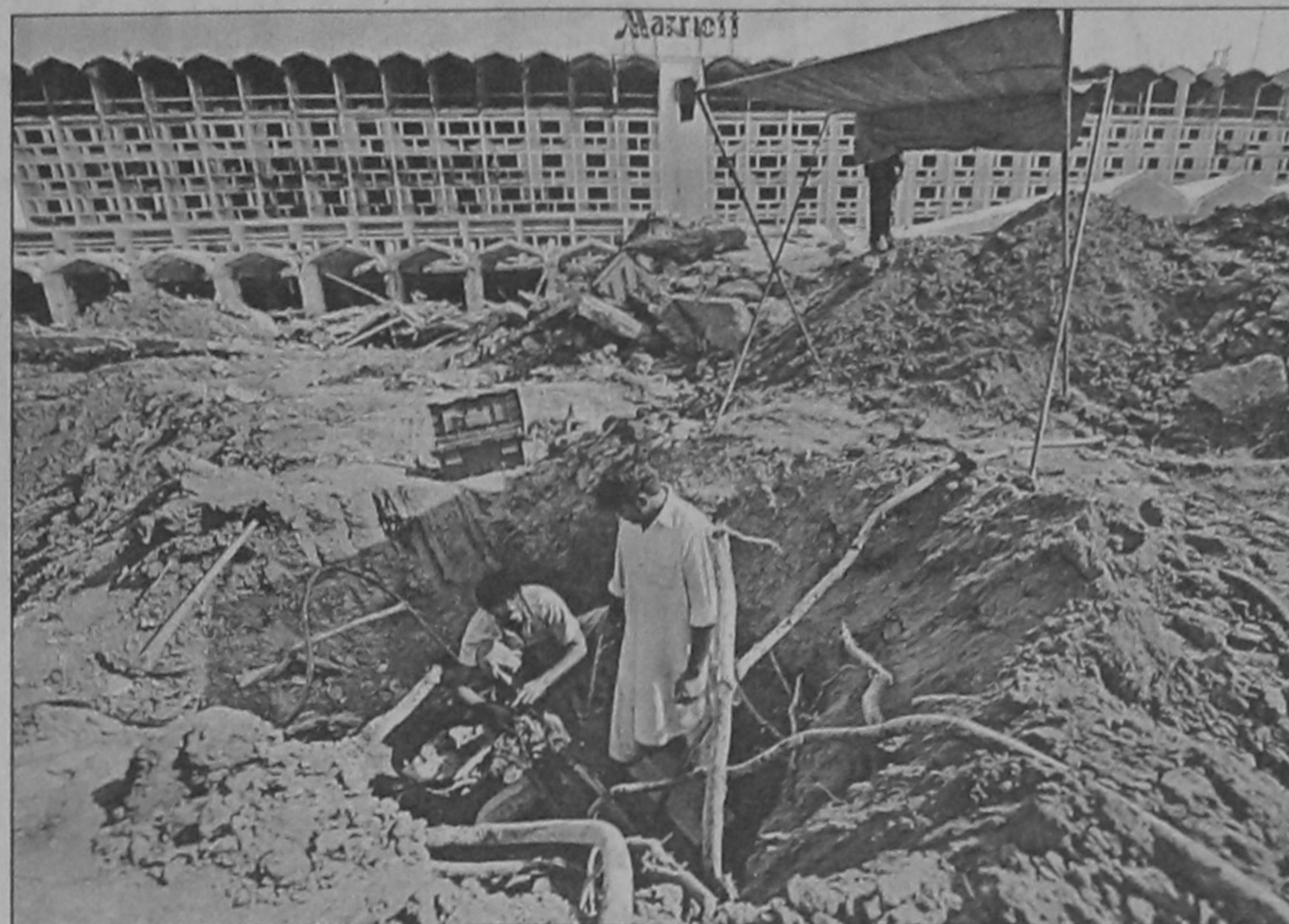
Pakistani workers repair telephone cables in front of the devastated Marriott Hotel in Islamabad yesterday, three days after a suicide attack. British Airways has cancelled all flights to the Pakistani capital Islamabad for an indefinite period amid security concerns after the bombing of the Marriott hotel, the airline said.
