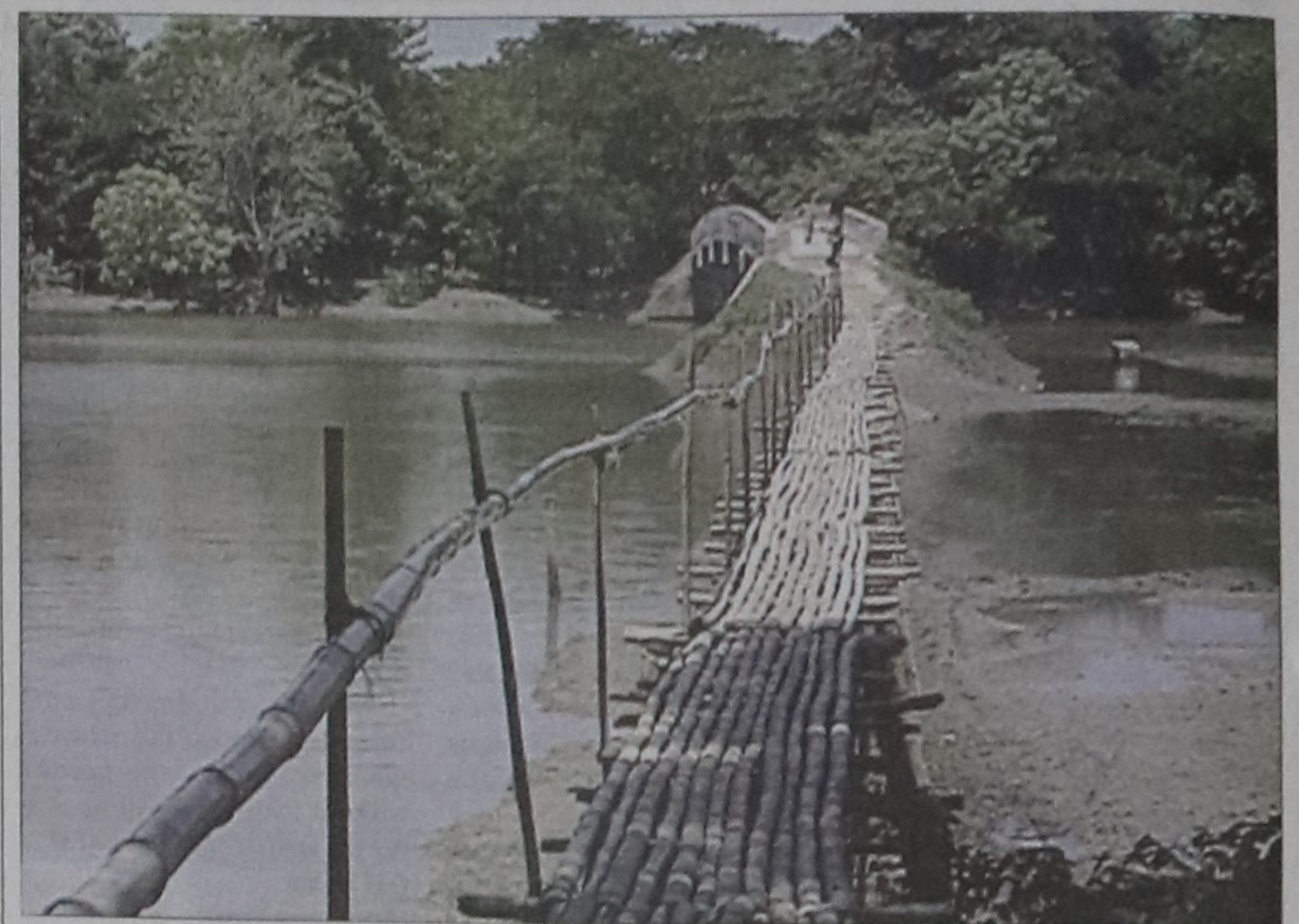
ACT OF CALLOUSNESS AND FUND EMBEZZLEMENT: But for the long bamboo-made structure made by locals, the Tk 11 lakh bridge on Parla-Telagati road across Mogra River in Netrakona would remain useless after one year of construction as the approach road is yet to be complete.
