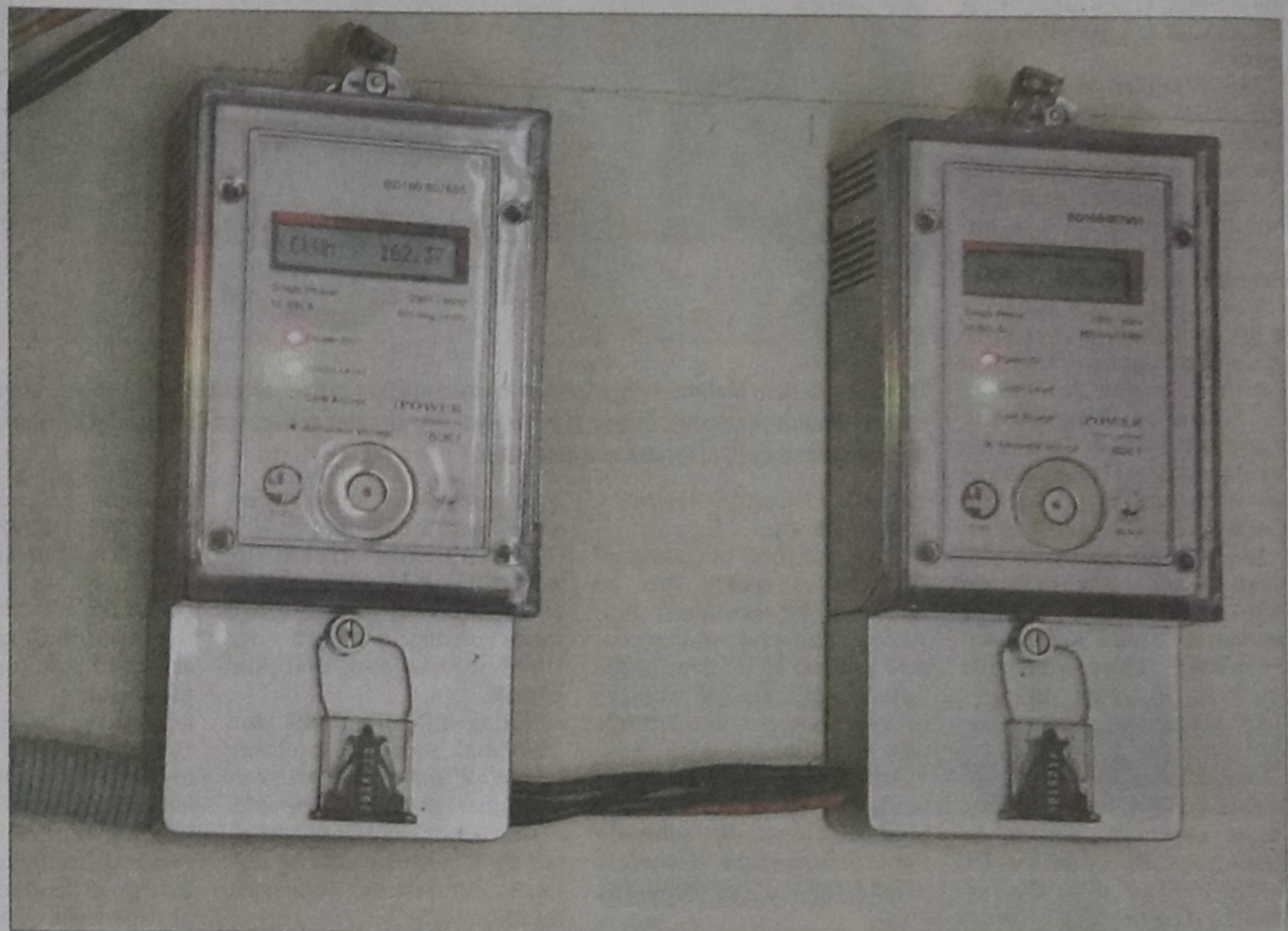
Two prepaid meters are installed in a house in Uttara.
