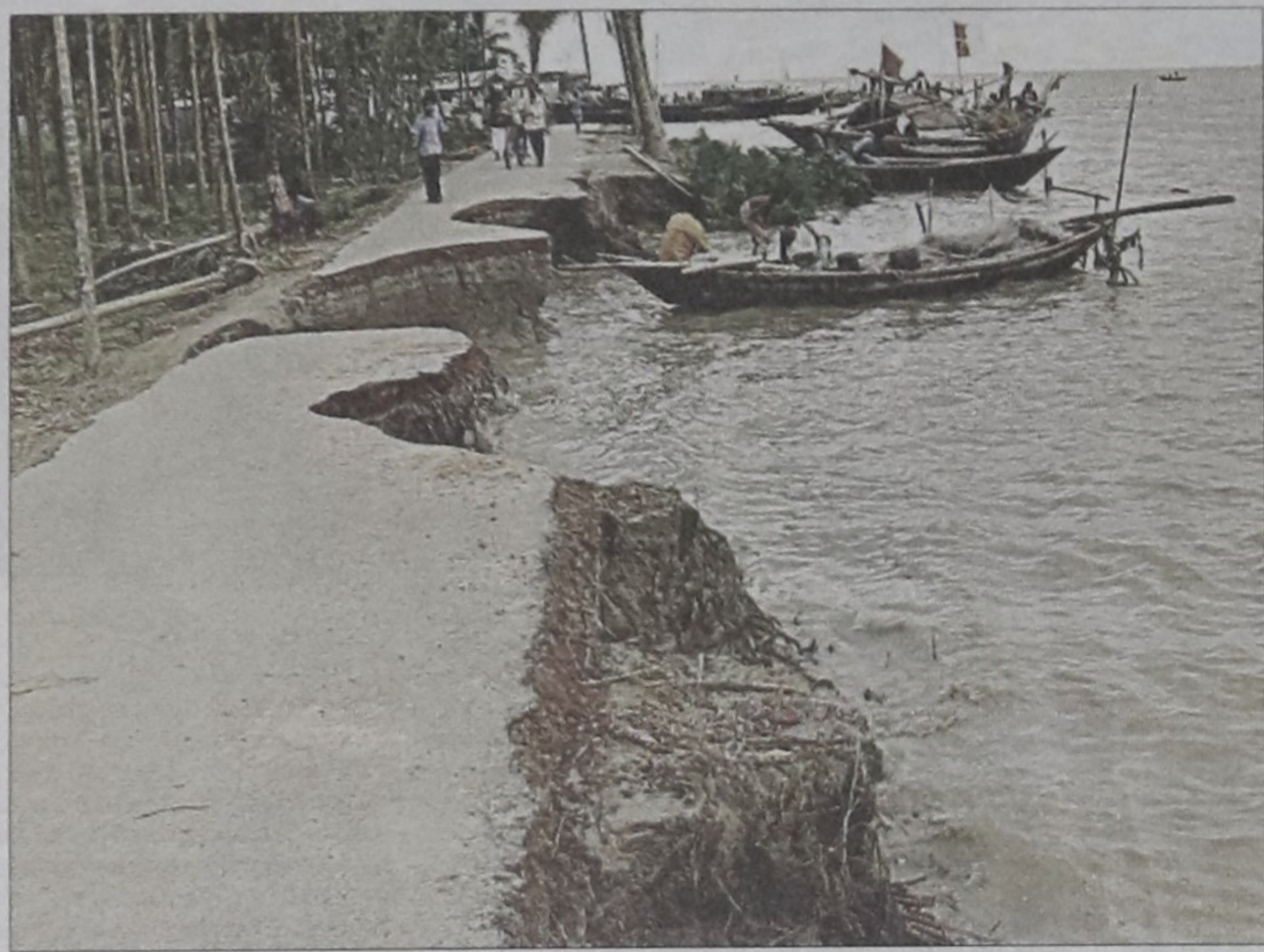
ROAD COMMUNICATION IN A LARGE PORTION OF HAIMCHAR UPAZILA IN CHANDPUR DISTRICT HAS BEEN VIRTUALLY CUT WITH EROSION TAKING A SERIOUS TURN IN THE IRRIGATION PROJECT AREA OF THE UPAZILA.
