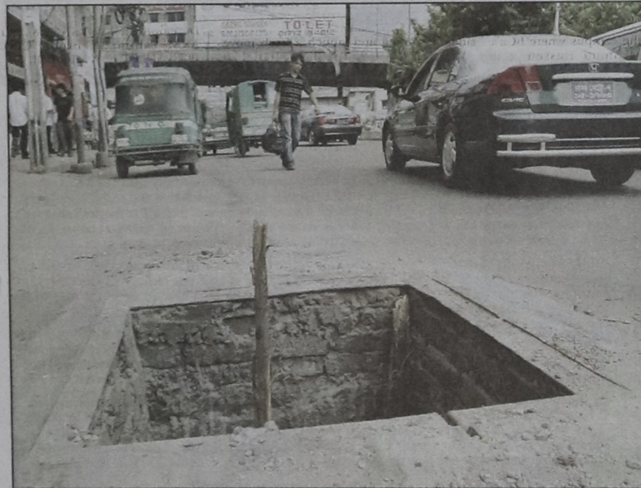
An open manhole on a road in front of Jalkhabar Hotel at Mohakhali in the city remains unrepaired for long, posing danger to pedestrians as well as passengers. The picture was taken yesterday.
