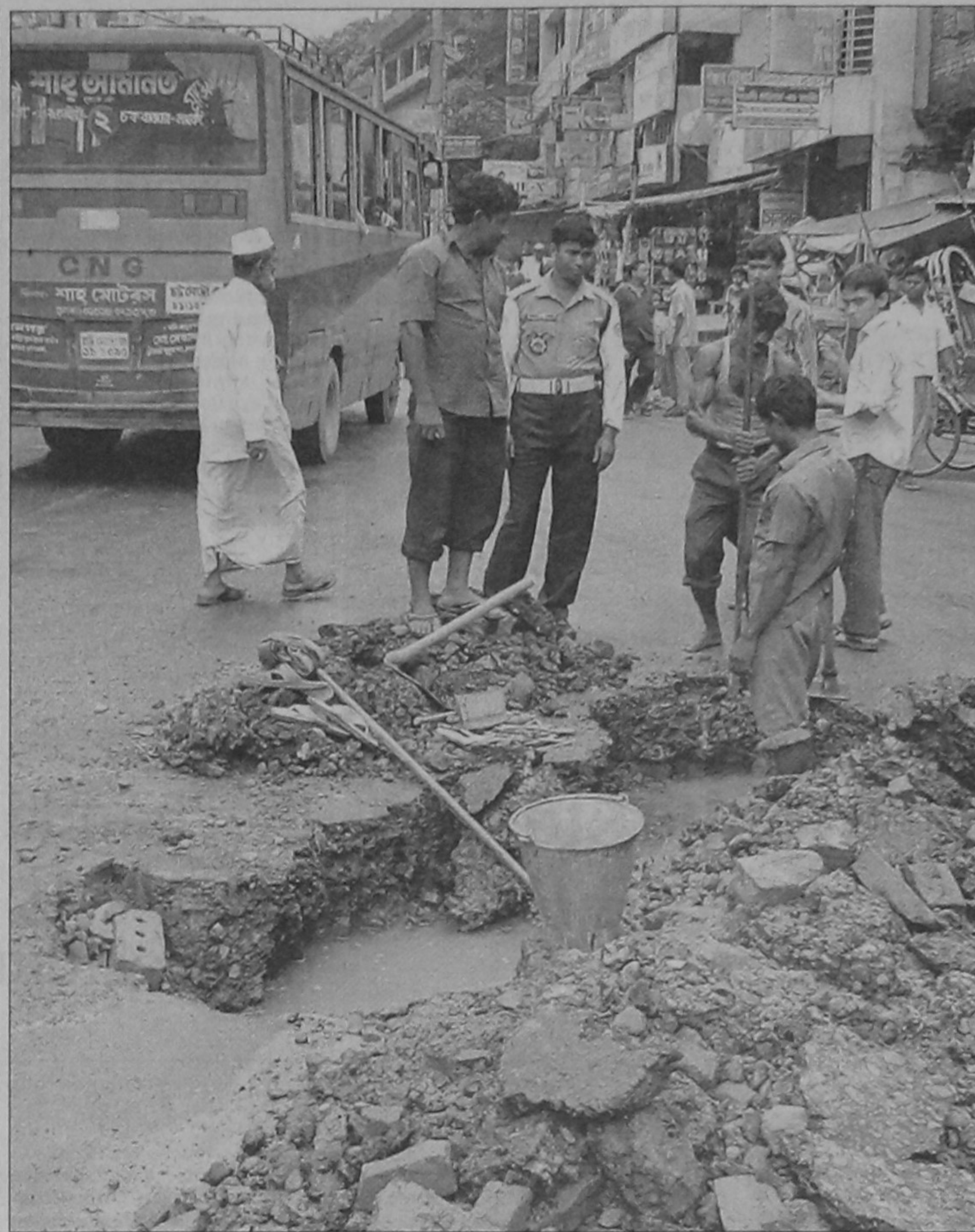
PHOTO: STAR Chittagong Wasa started digging in the middle of busy Anderkilla-Bakshir Hat intersection in the port city in order to repair a Wasa pipeline yesterday, adding to the suffering of the commuters and pedestrians in the rainy season.
