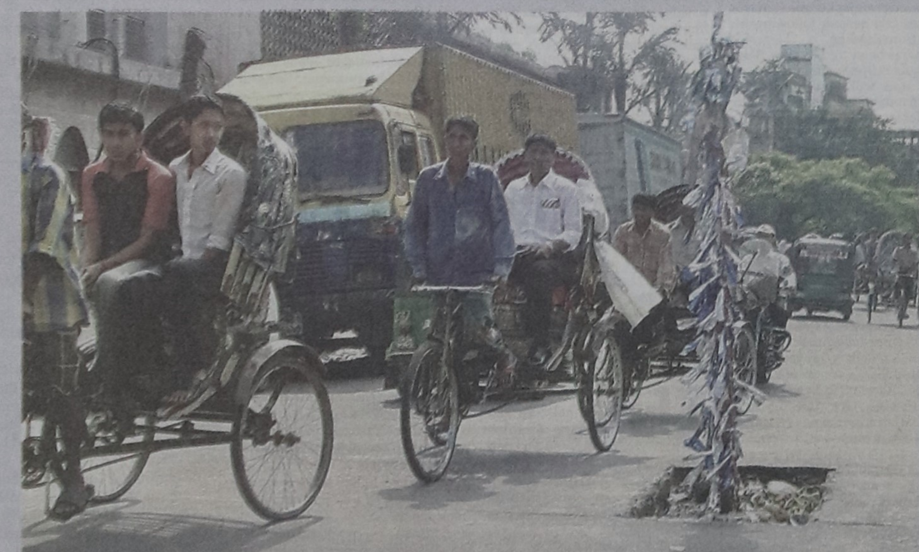
(Left) A concrete slab on a drain on the Commerce College Road in the city's busy Agrabad Area has been missing for around one month posing a danger to the pedestrians as well as vehicles. A local shopkeeper has set up a pole on the drain to make the people aware of the danger when the authorities concerned remained indifferent to the problem.
