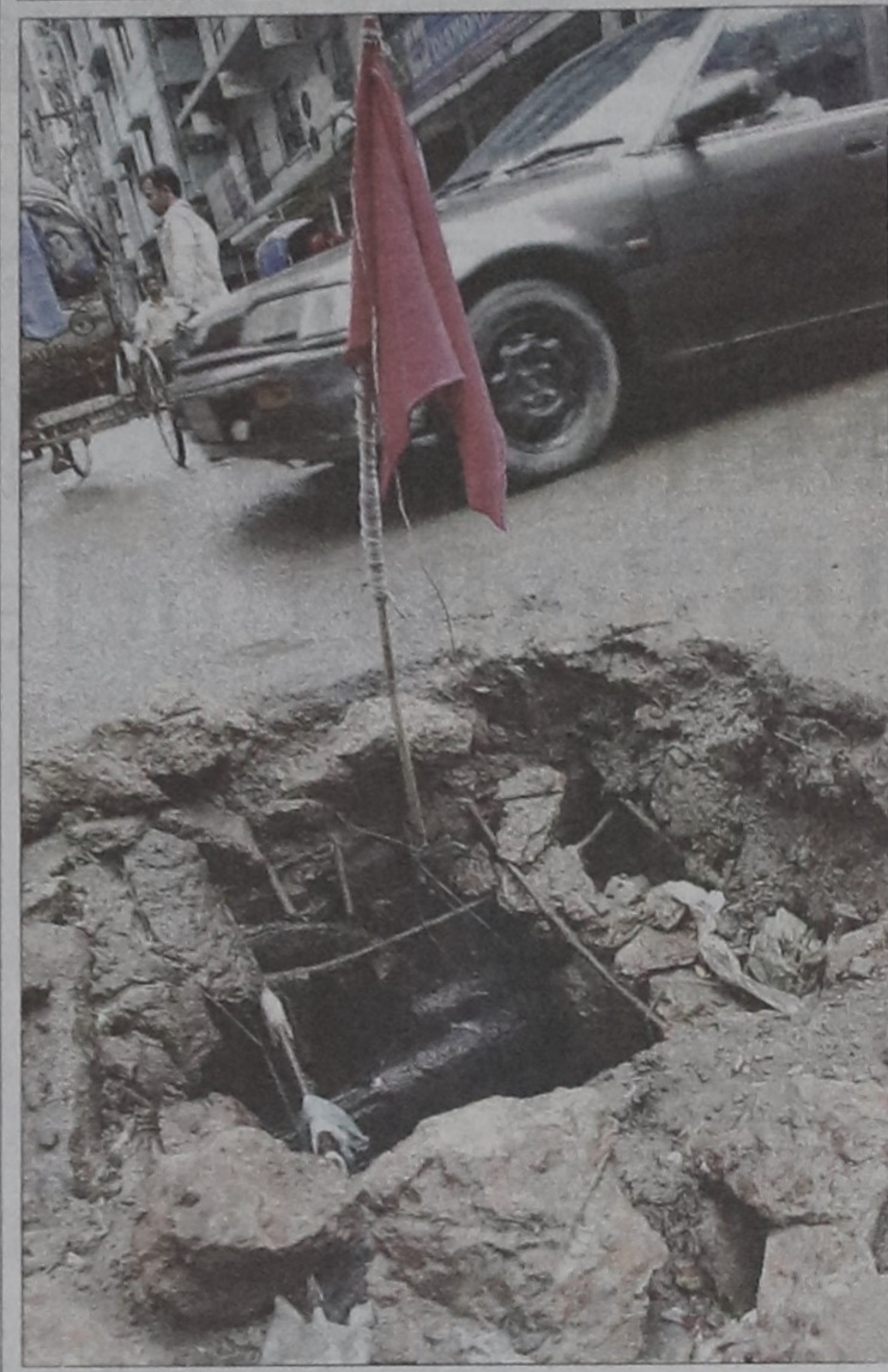
A broken manhole without cover on a road in Purana Paltan poses danger to pedestrians as well as passengers. Local people have put up a pole with red cloth to make passers-by aware of the danger. The photo was taken yesterday.
