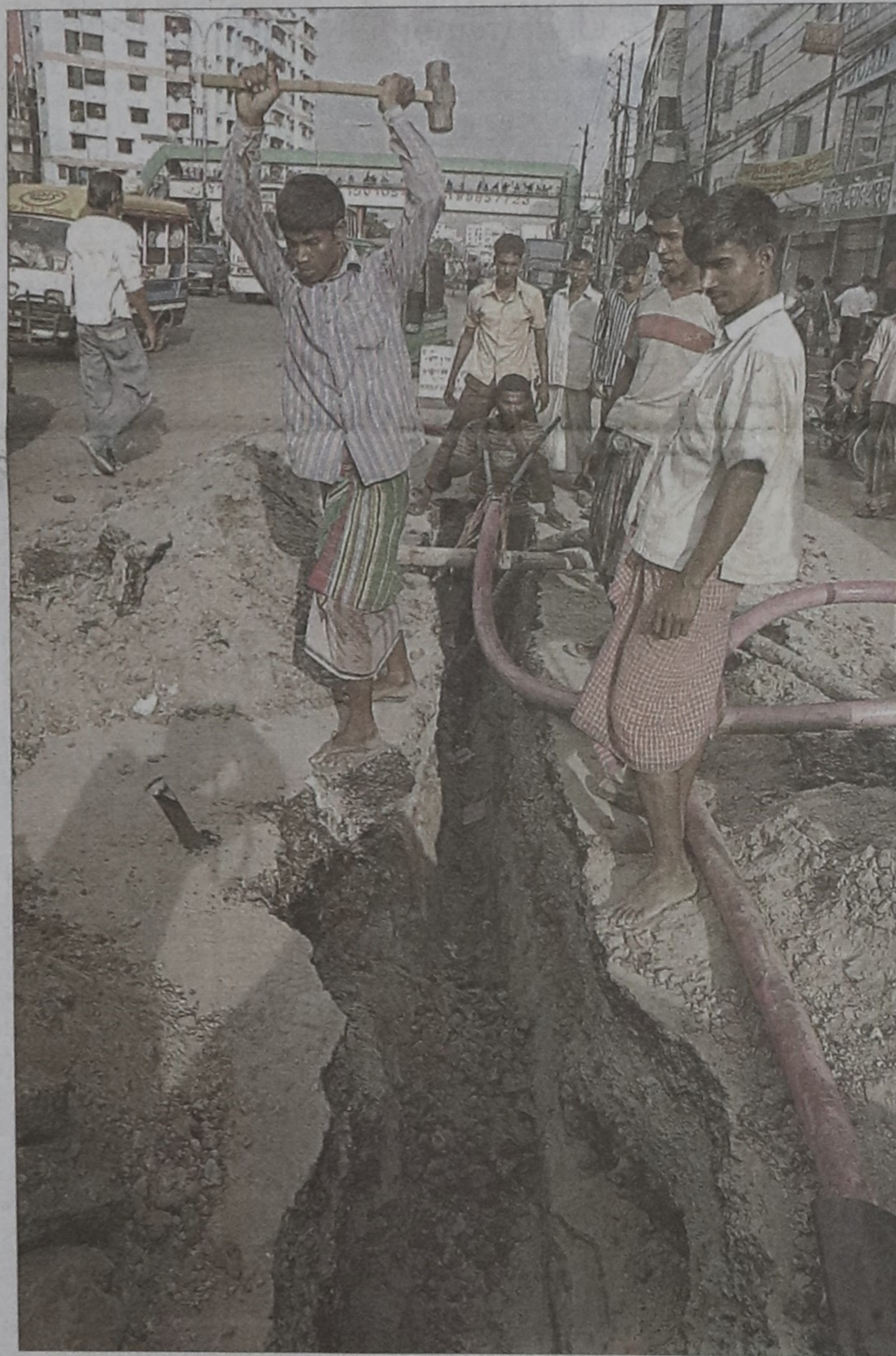
Dhaka Power Distribution Company digs a trench on Mirpur Road at Kalyanpur to work on a power cable ignoring the chief adviser's July 2 directive to stop road digging in the rainy season.
