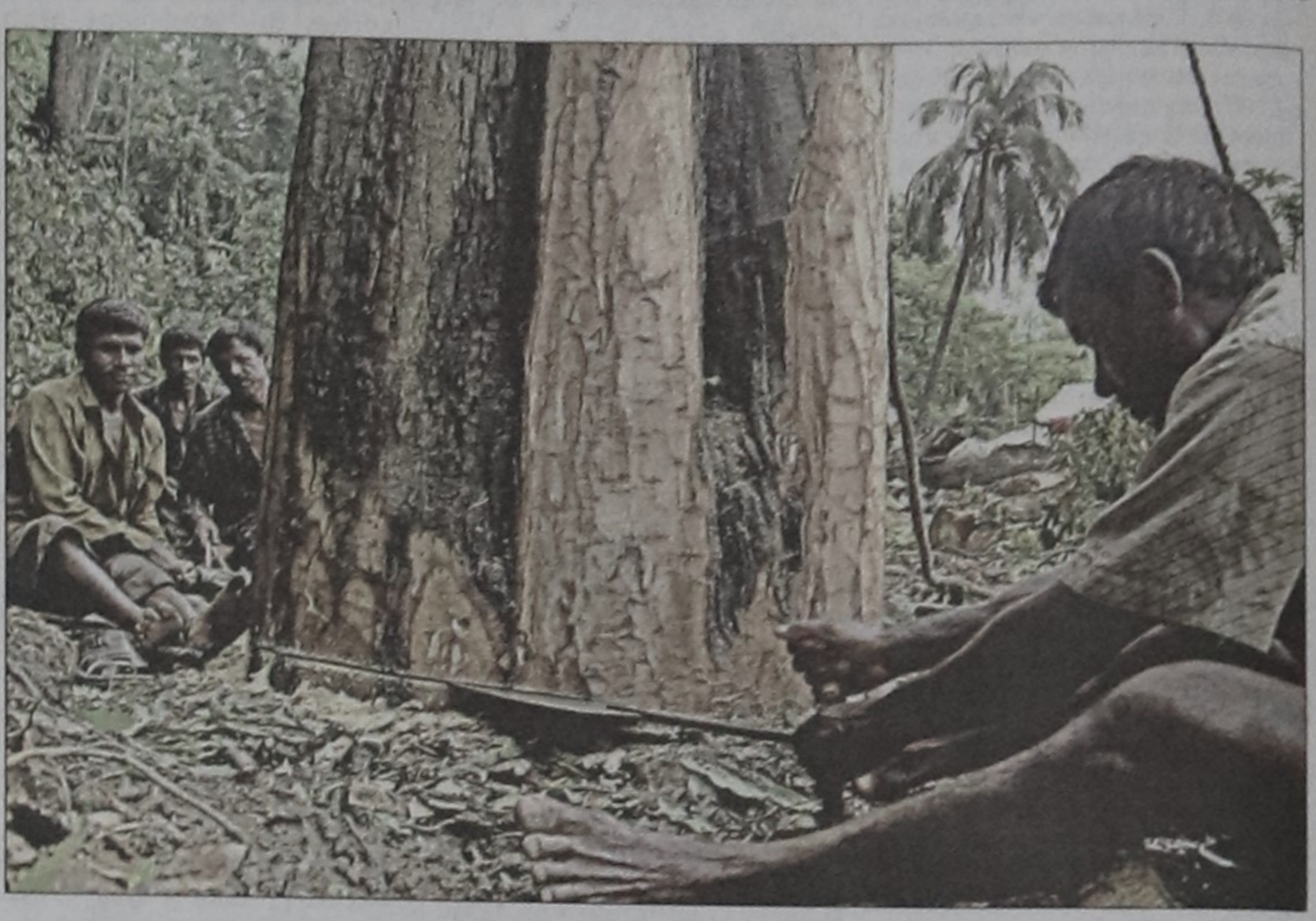
Trees are being felled on Jagannath Hall premises at Dhaka University yesterday to make space for an extension building to accommodate increasing students.
