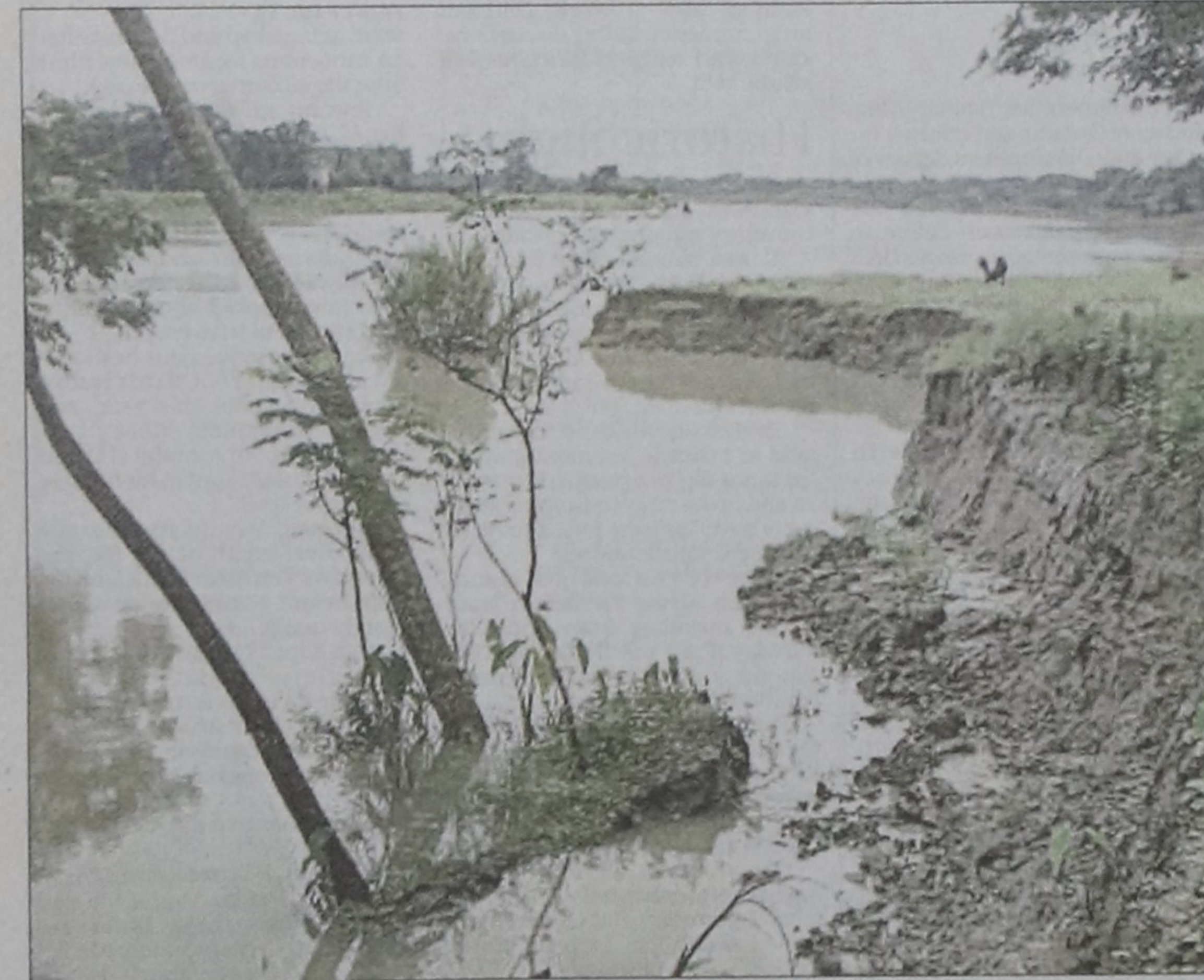
Severe erosion by the Kushiara at Shenpotir Chawk point in Sylhet. Bangladesh loses thousands acres of land in the process to India as the other side of the river automatically turns into its (Indian) territory.
