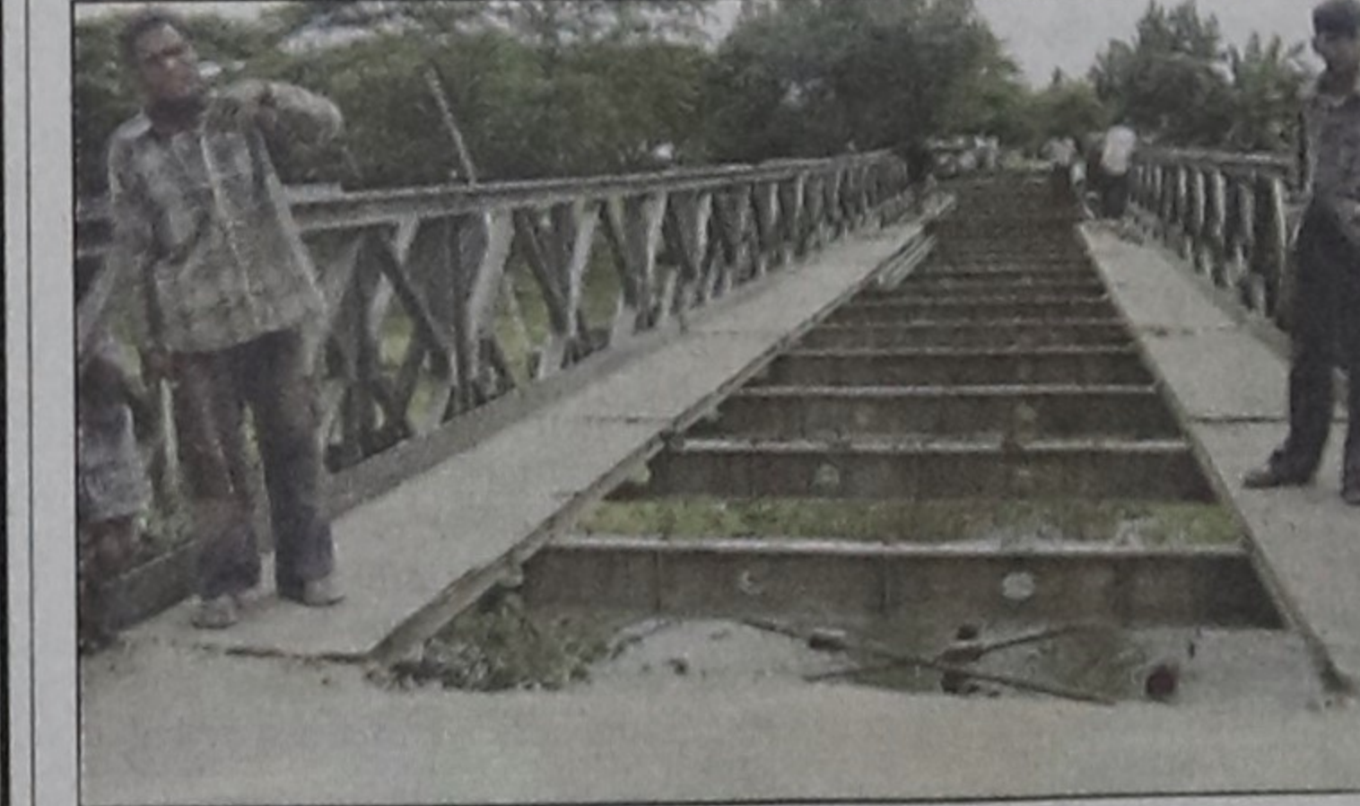
Expired 14 years ago, Rashidabad baily bridge at Kishoreganj town is being disassembled without making any alternative arrangement.
