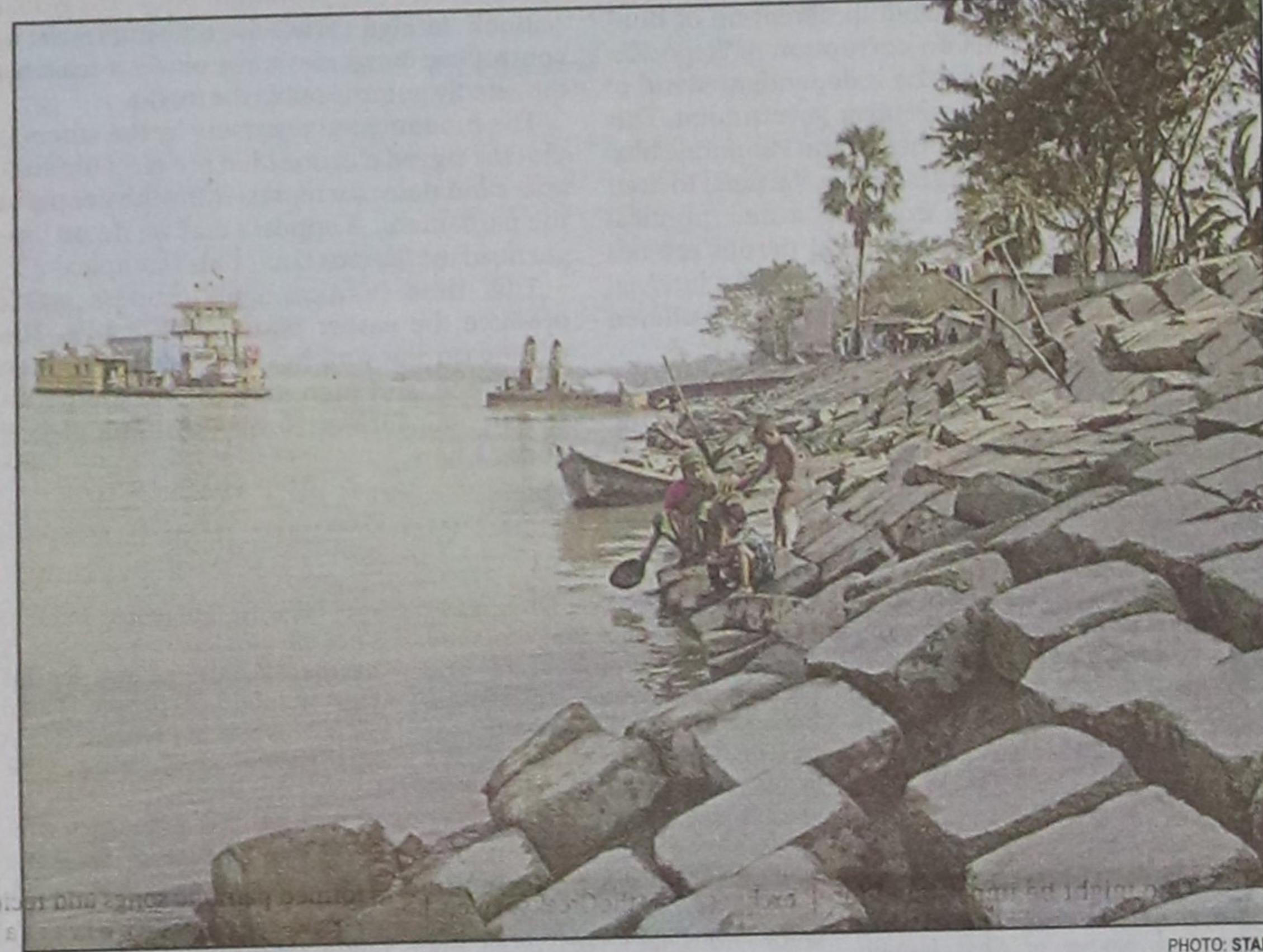
Patuakhali-Barisal Highway at Dumki is threatened as Water Development Board's concrete slab protection embankment on Paira River is being battered by waves.
