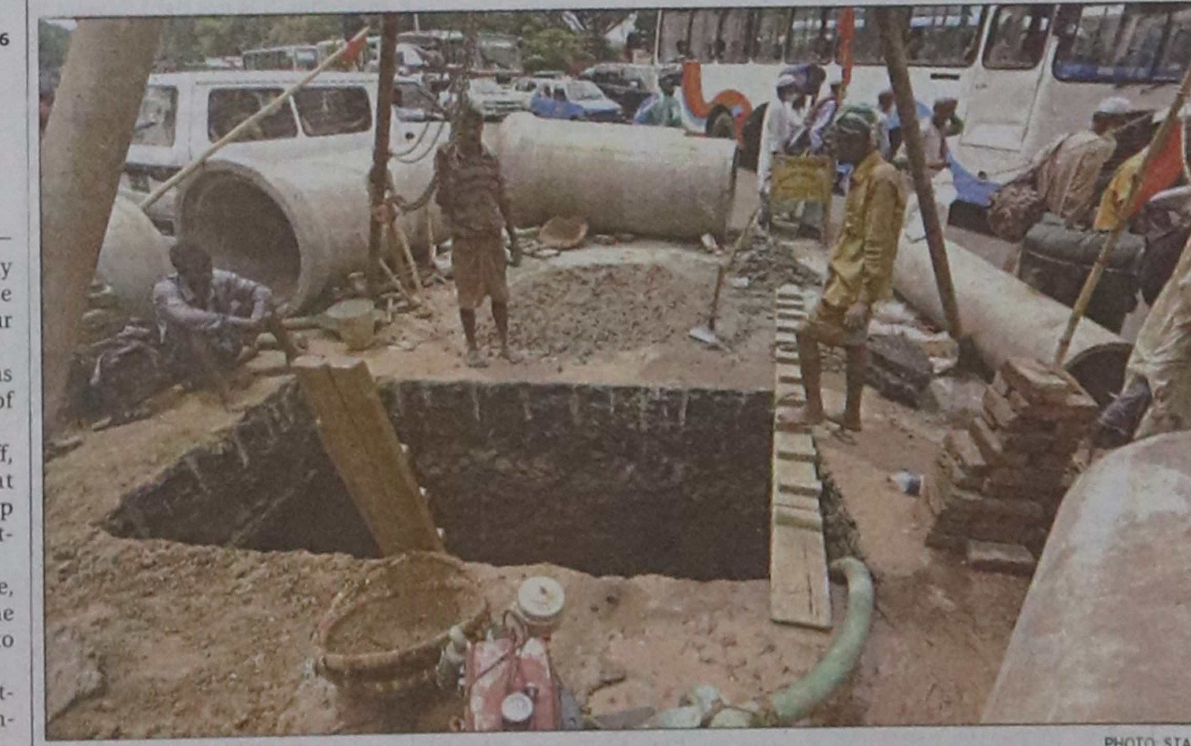
Traffic grinds to a halt near Matshya Bhaban in the capital yesterday as Dhaka Wasa installs drainage pipes, narrowing down the usable road.
