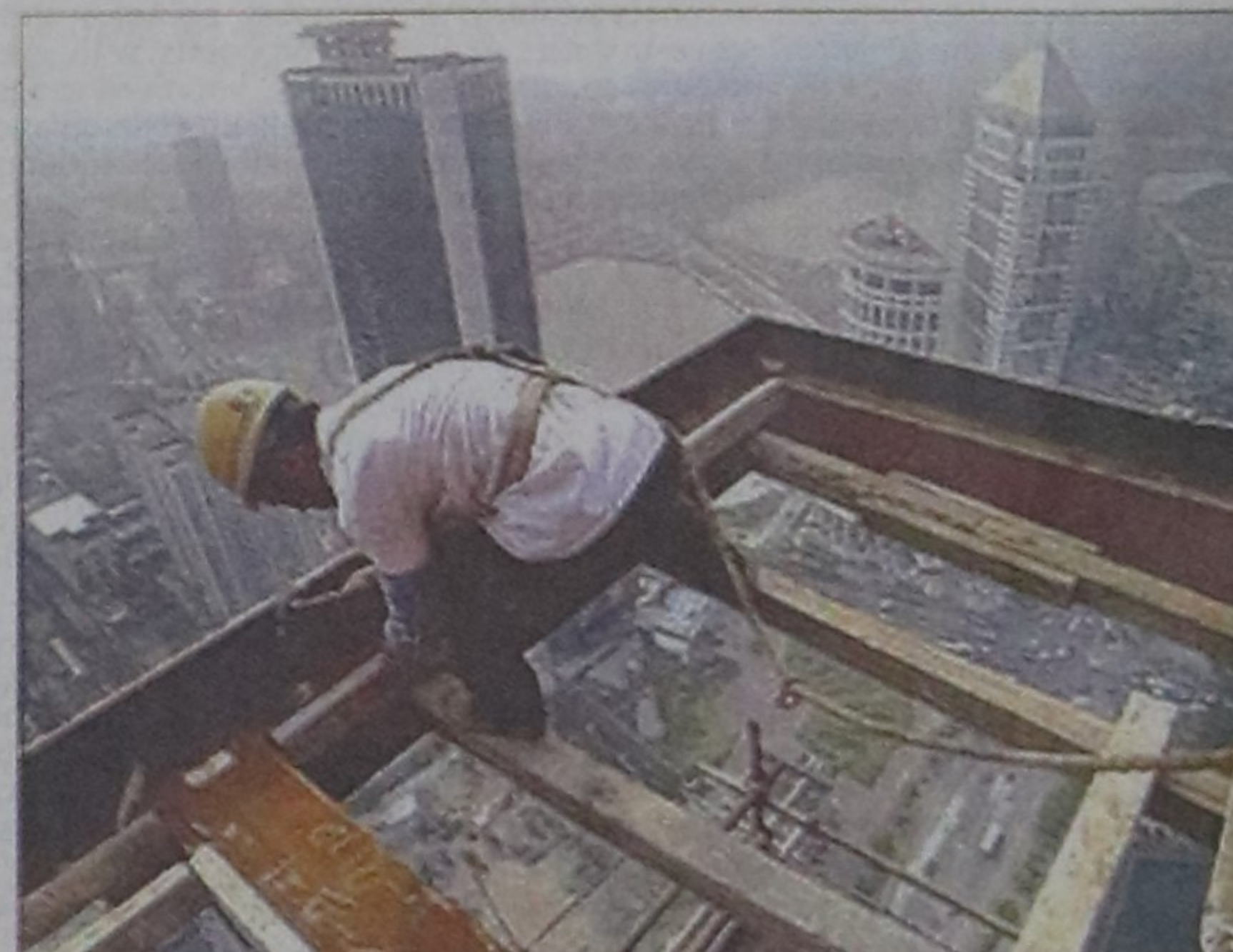
A Chinese construction worker goes about his work on a platform hanging over a skyscraper building site in Wuhan. China's economy can maintain a steady growth above 8 percent for a relatively long period because of a stable society, a vast market and ample capital.
