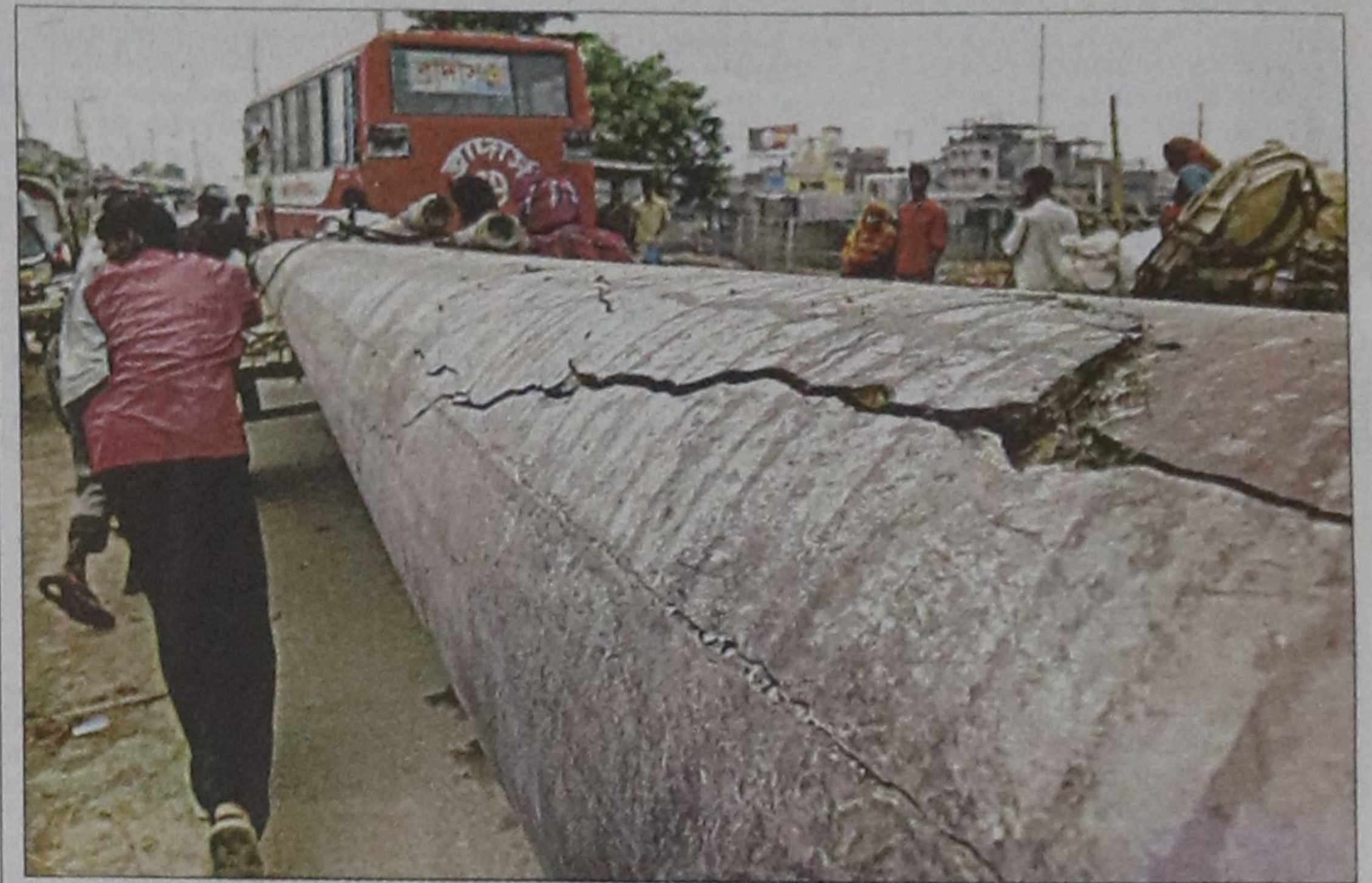
A concrete electric pole with cracks is being taken to Lalbagh in the capital on a pushcart yesterday for using in the electricity supply system of the area.
