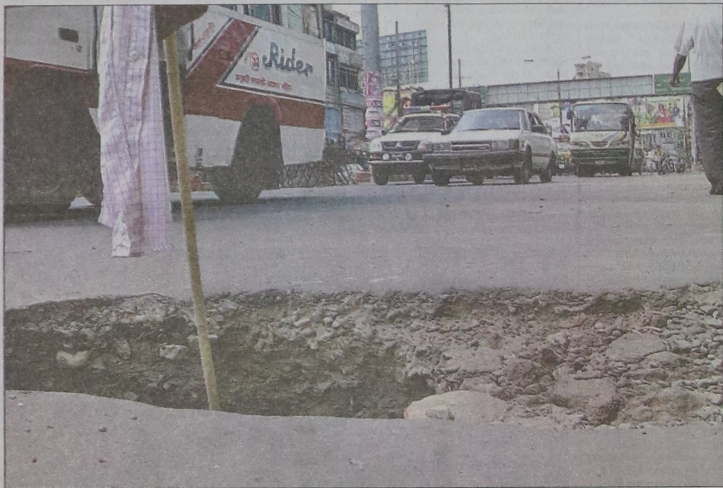
This large hole at Chowmuhoni Intersection on the ever-busy Agrabad Sheikh Mujib Road may cause accident any time. The photo was taken on Monday.
