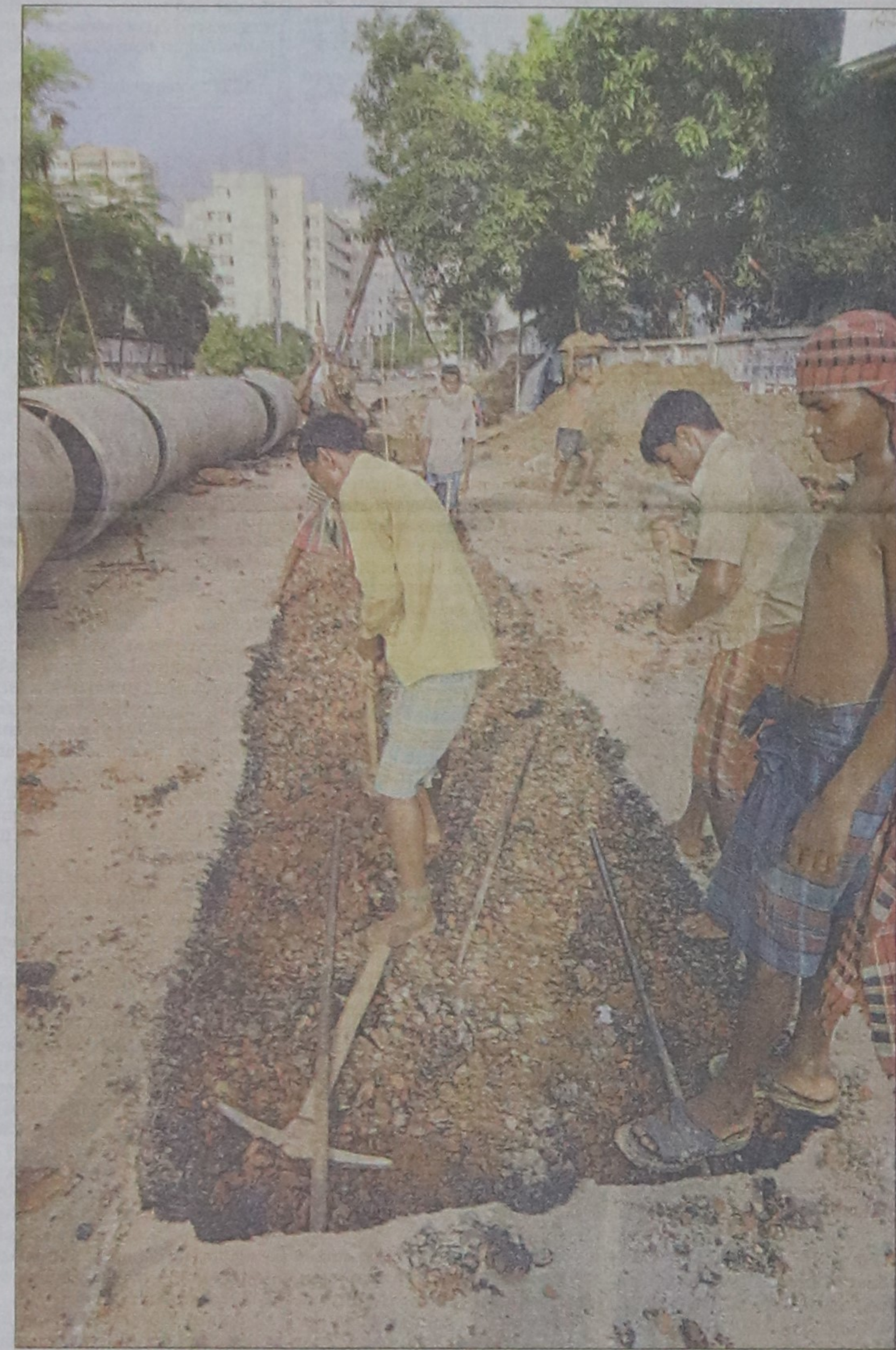
Dhaka Wasa tears off a large section of tarmac near Matshya Bhaban intersection in the capital to install drainage pipes under the street. The photo was taken yesterday.
