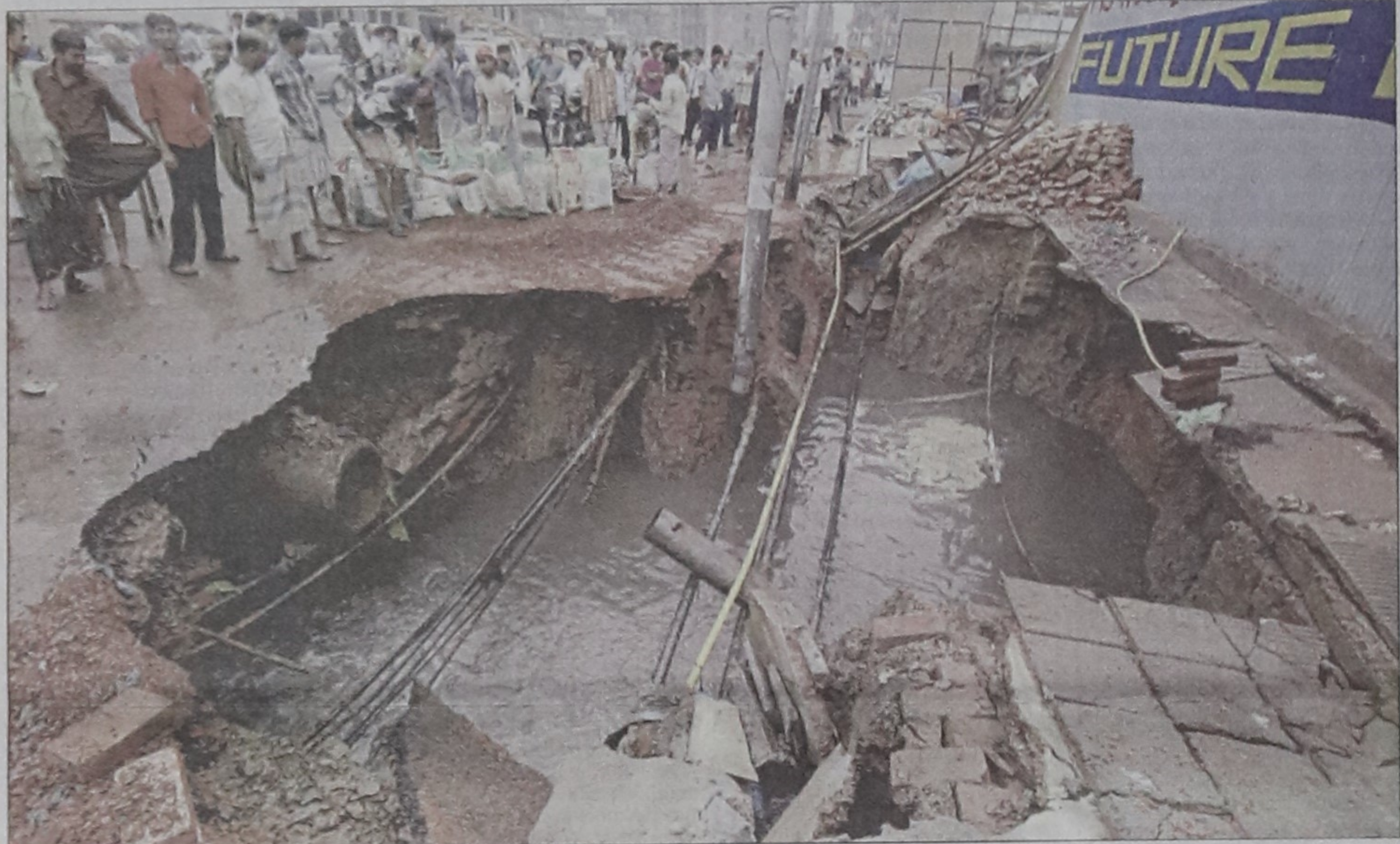
A section of the Kakrail-Shantinagar road along with the pavement subsides during yesterday's heavy rain in the capital. A large hole has been dug on the other side of the tin fence to construct the foundation of a building.
