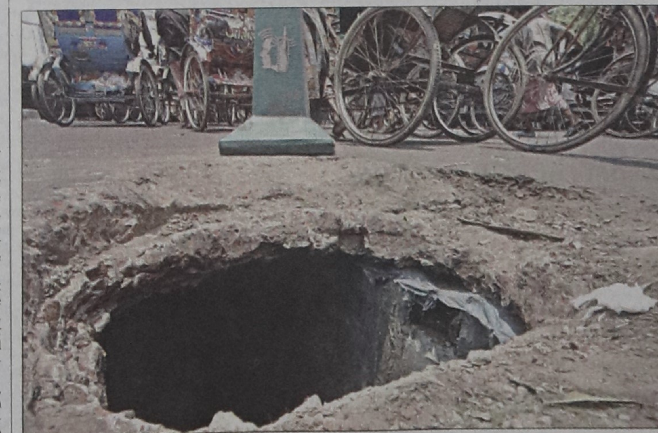
A broken manhole on a street in Bijoy Nagar in the capital puts vehicles and people at risk. The photo was taken yesterday.
