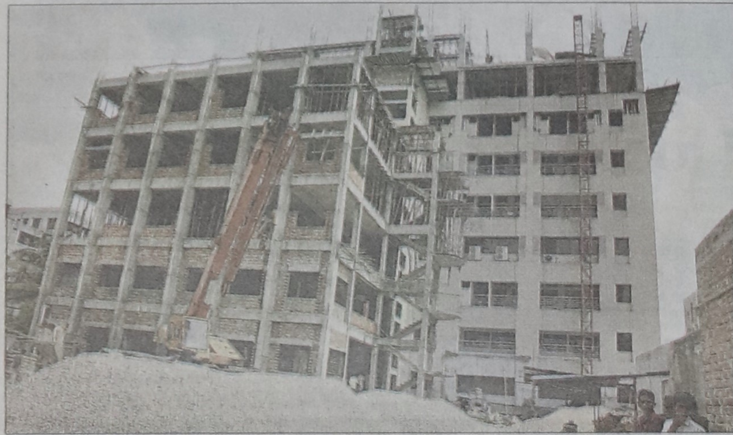
The under construction 150-bed building of national cancer institute and the unused CT scan machine.
