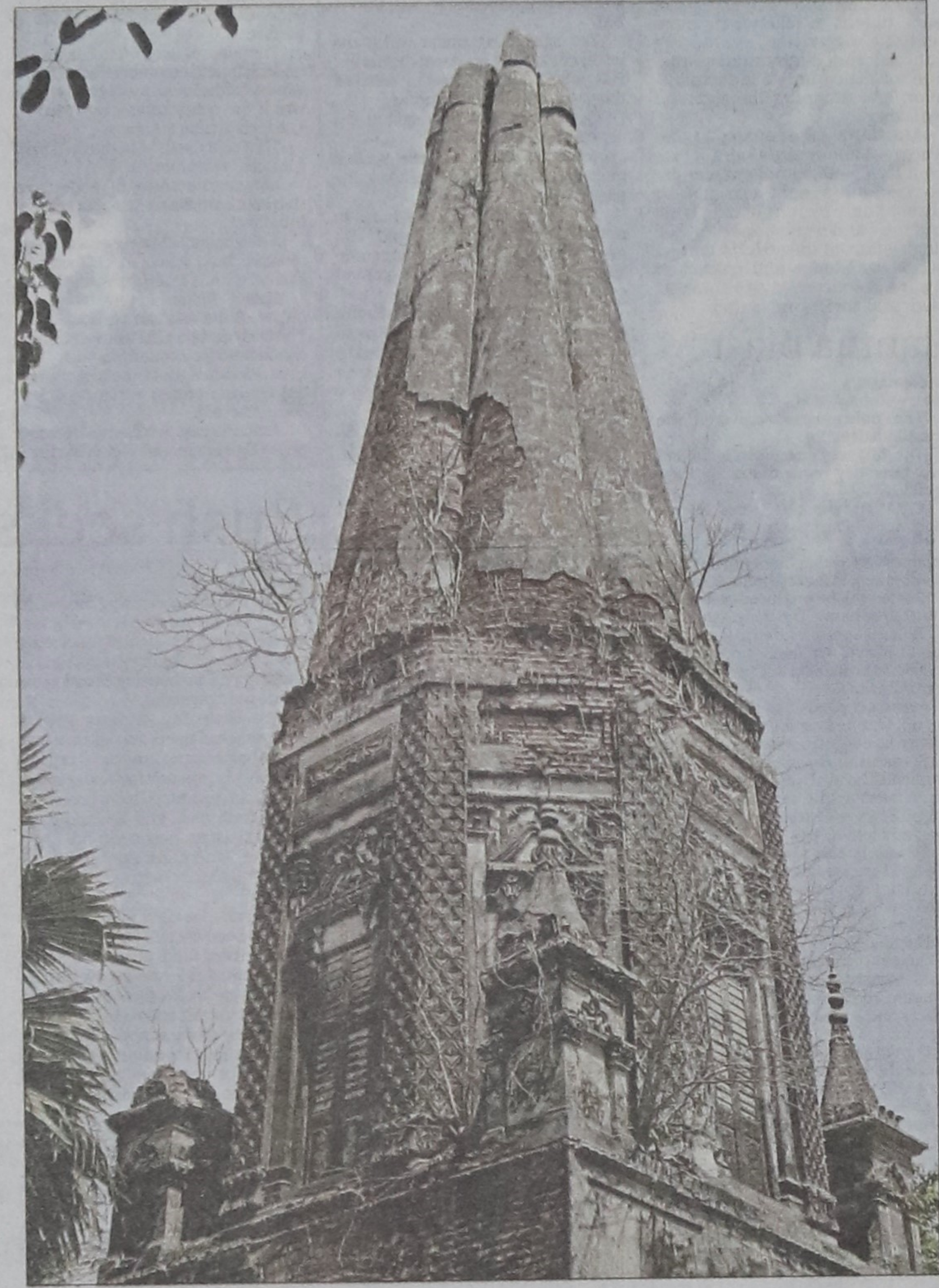
The 127-year-old Uday Tara Chowdhurani Matha in Nagarpur upazila of Tangail lies in a dilapidated condition with most of its plaster fallen off and plants growing through cracks.
