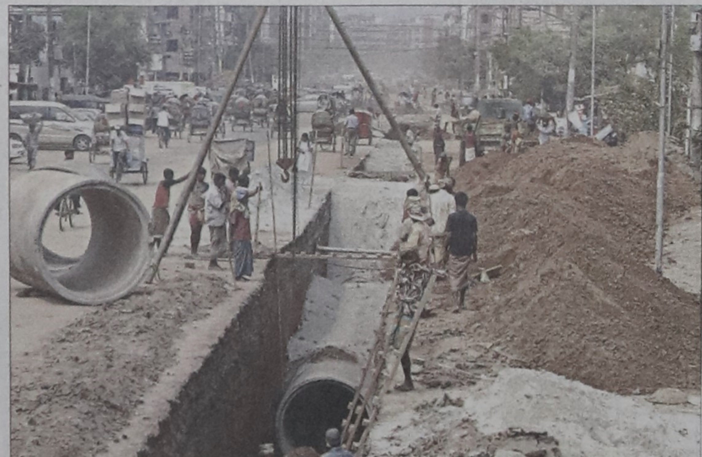
The work of the 25-kilometre drainage goes on at Uttara town. Land digging for the project in the area is causing serious traffic congestion at some points.
