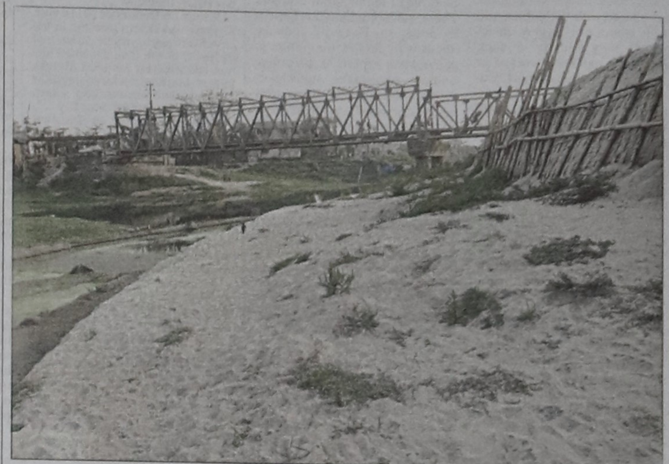
The Satarkul canal in Badda in the capital falls victim to land grabbers narrowing down the width of the canal considerably. The photo was taken yesterday.
